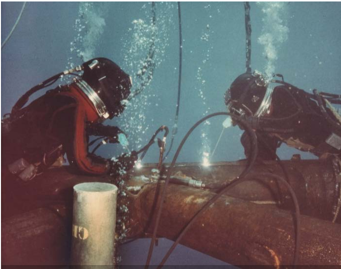
Two divers completing an underwater welding job on a platform, Whitey Grubbs (2002)
