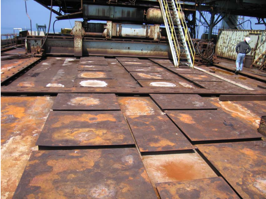
Figure 20. Drilling deck showing well slots with covers.
