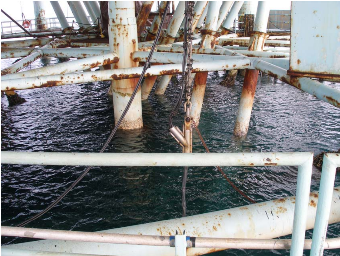
Figure 23. Open area at 15-foot deck level showing anode cable.
