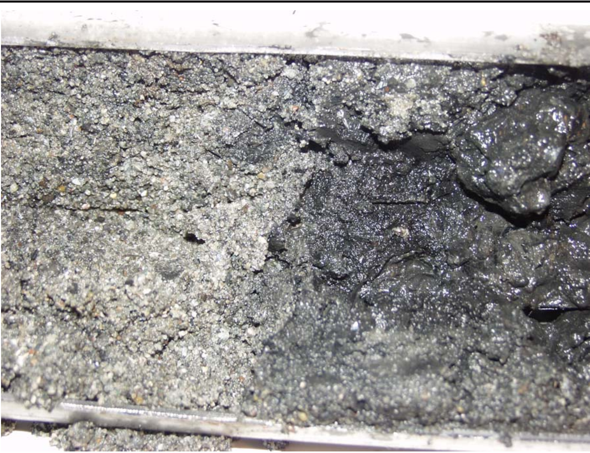
Gina – 1: Depth Interval; 1.4 feet (close up of upper sand layer and product-infused area).
