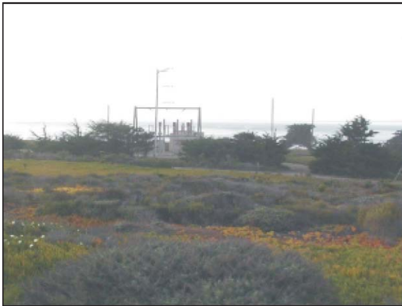
Figures 5.13-3: View of Surf Substation (View Position 2) (View of Surf Substation looking west from the west end of Ocean Avenue. The low vegetation is in the foreground, the substation is in the mid-ground and the ocean is in the background.)
