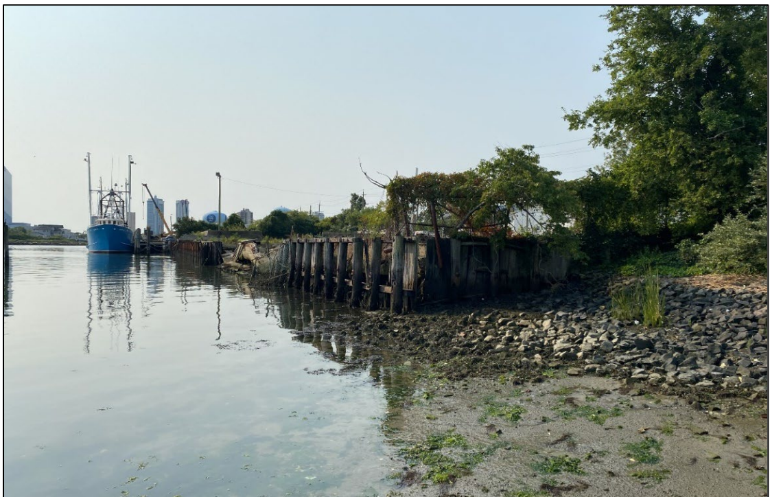
Photograph 3. Overview of partially collapsed wood and concrete bulkhead facing the marina. View to the south.
