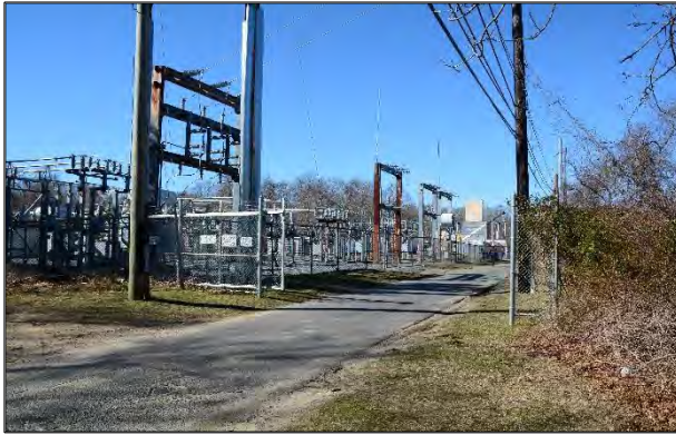
Inset 8 – LIPA Substation
