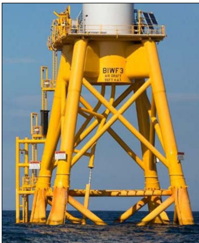
Figure 3-2 Photo of air draft marking on a wind turbine
