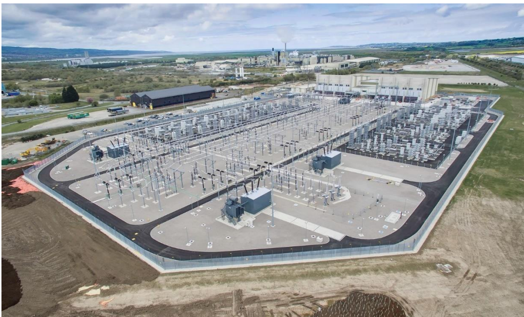
Figure 3 - Example LCC Converter Station (Western Link, 2200MW)
