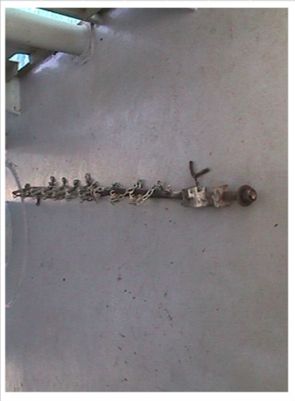
Fallen Pipe Rack Finger
