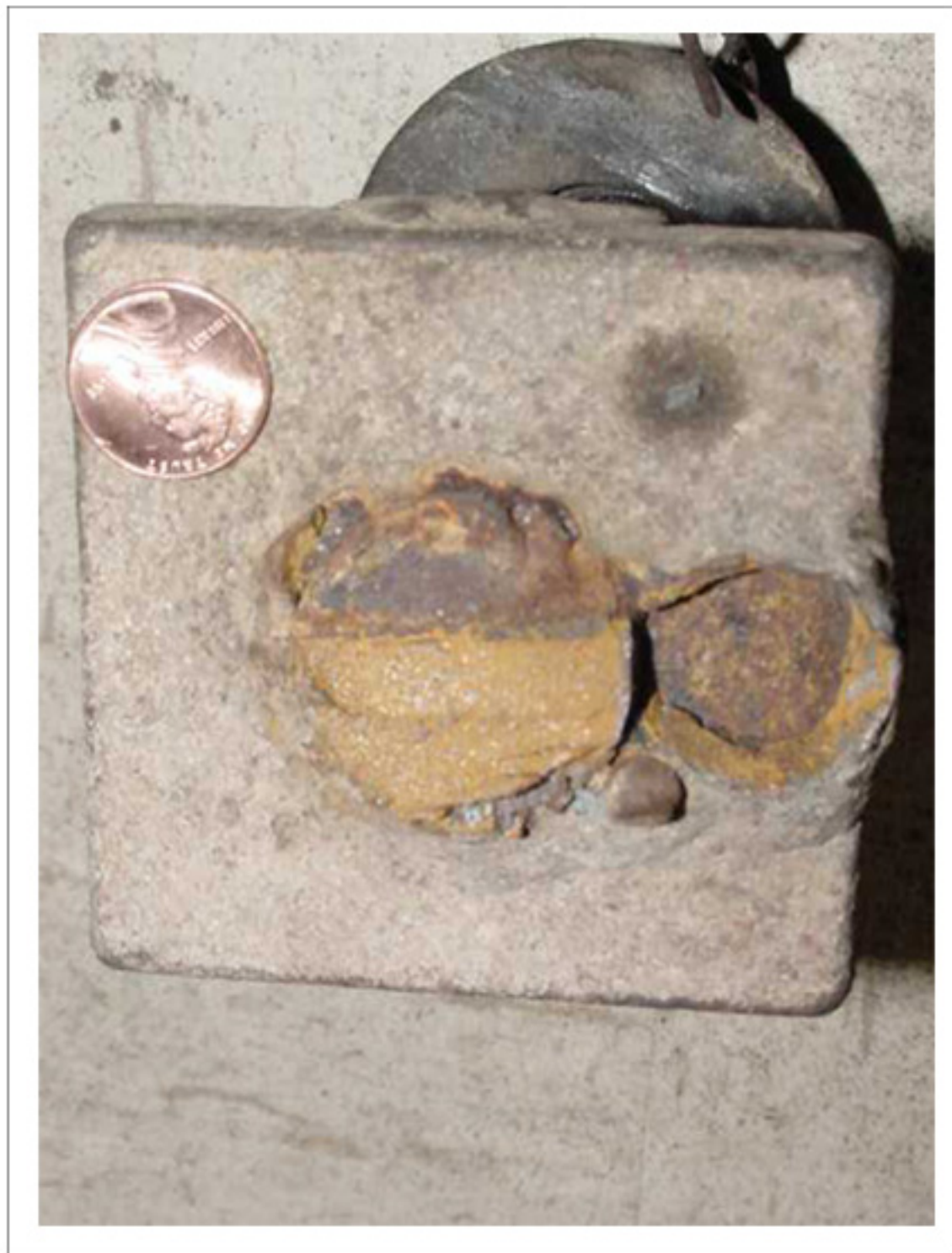
Base-End of the Broken Pipe Rack Finger Removed from the Derrick after the Accident.
