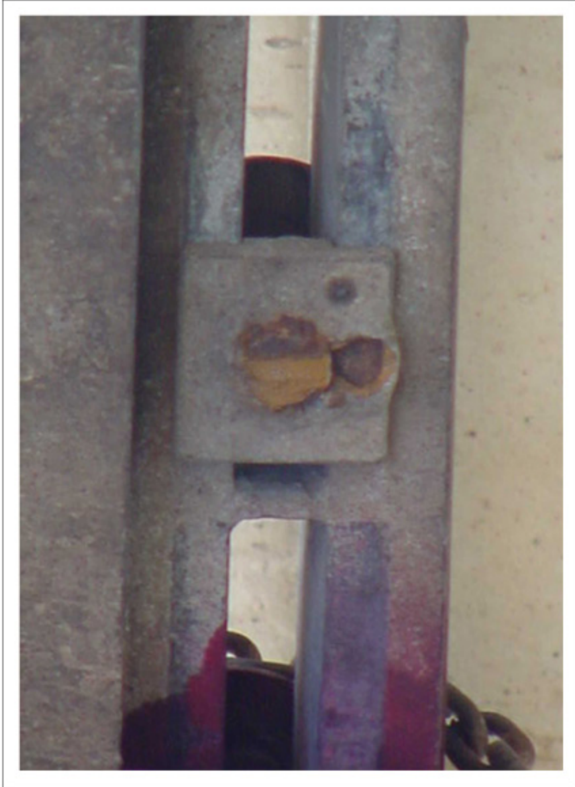
Base-End of Broken Pipe Rack Finger still Attached to Derrick after the Accident
