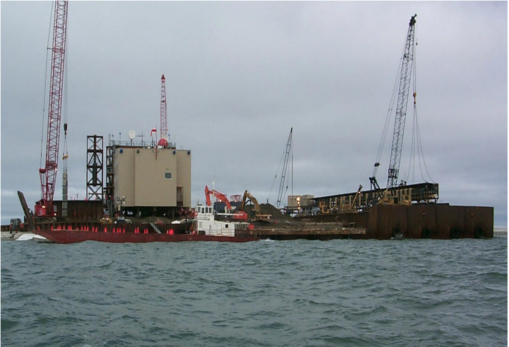
Fig. 3 Module on Northstar Island, August 2000. Crane at left hoisting concrete blocks linked together into a concrete mat. The mat is to be placed on Island slope to protect against wave and ice action.
