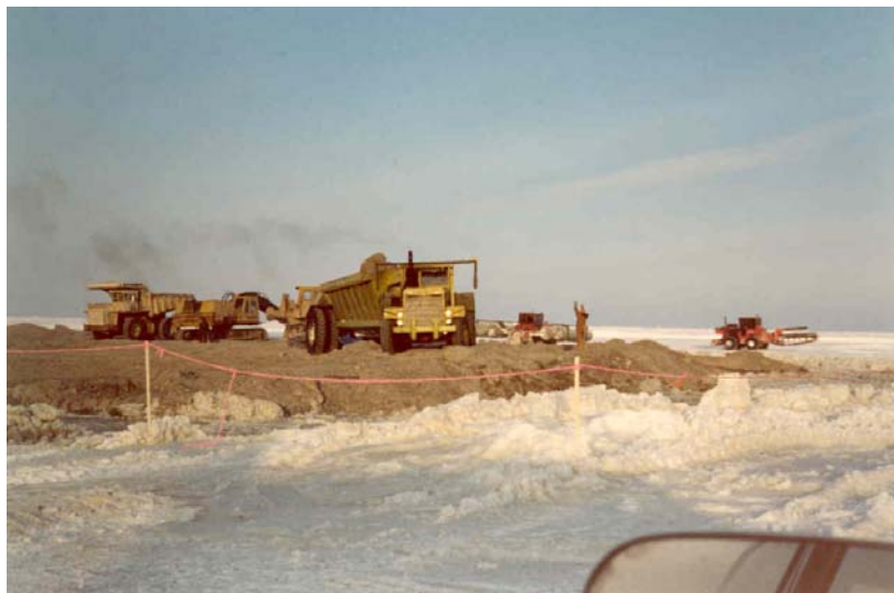
After surfacing of the gravel, trucks drive onto the new island to unload
