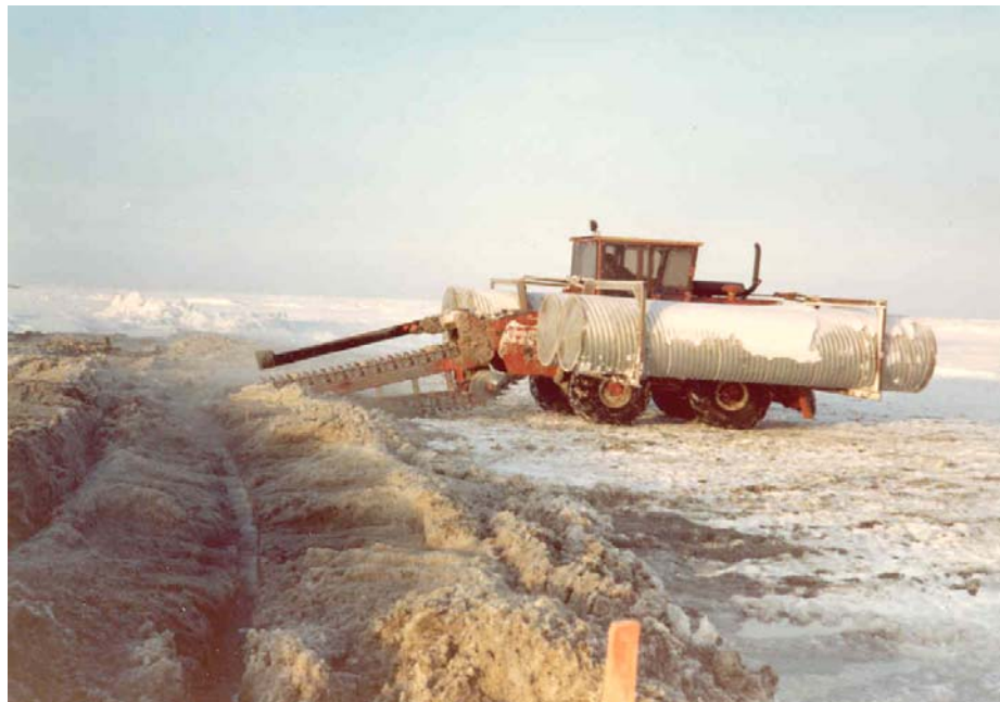
Widening of the ice hole with a Ditchwitch cutting machine (equipped for buoyancy tanks in case of break-in)
