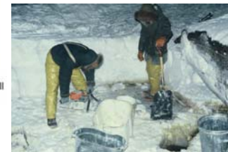
Diesel spill under snow Photo: D. Dickins
