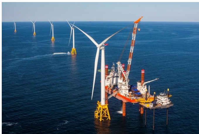
Block Island Wind Farm (Deepwater Wind)
