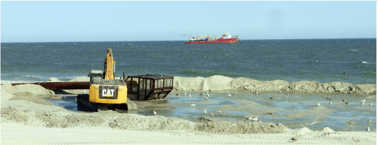
Dredge Ship Liberty Island transports dredged sand closer to shore for the pump-out at Long Beach Island, NJ. Photo by Marjorie Weisskohl, BOEM.
