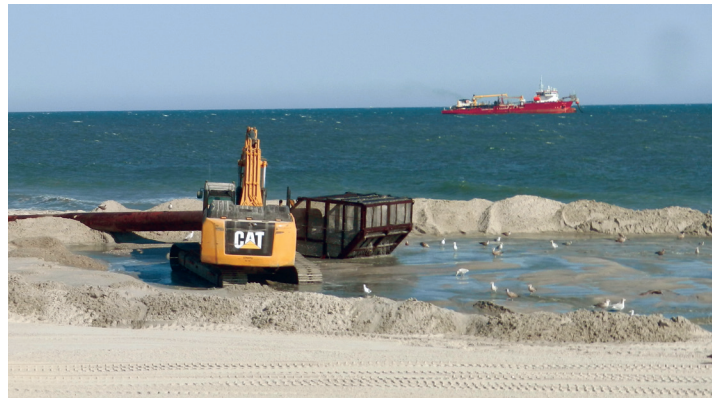
Beach construction underway at Long Beach Island, Oct. 2015. Photo by Marjorie Weisskohl, BOEM
