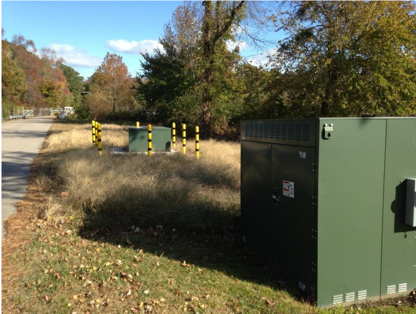
View east on S. Birdneck Rd. toward Dam Neck. Note existing switch cabinet.
