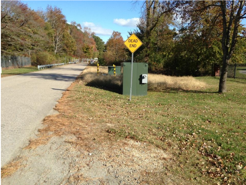
View of existing switch cabinet on S. Birdneck Rd.
