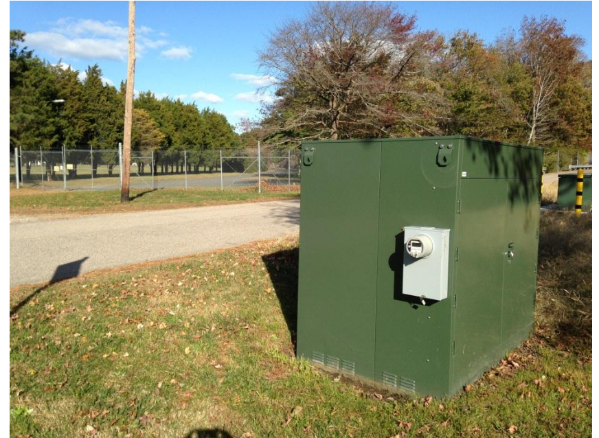
View north across S. Birdneck Rd from the existing switch cabinet toward the proposed interconnect station area.
