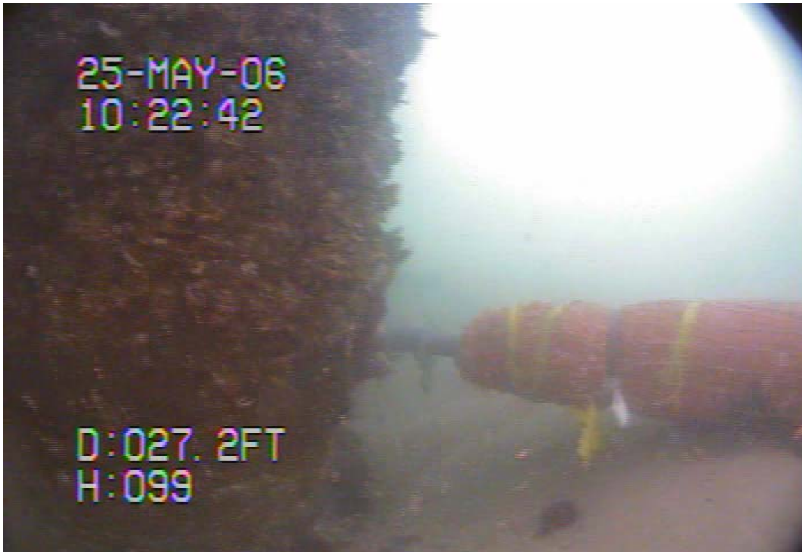
12. Mat on bottom ready for installation and scour at base of Southeast pile
