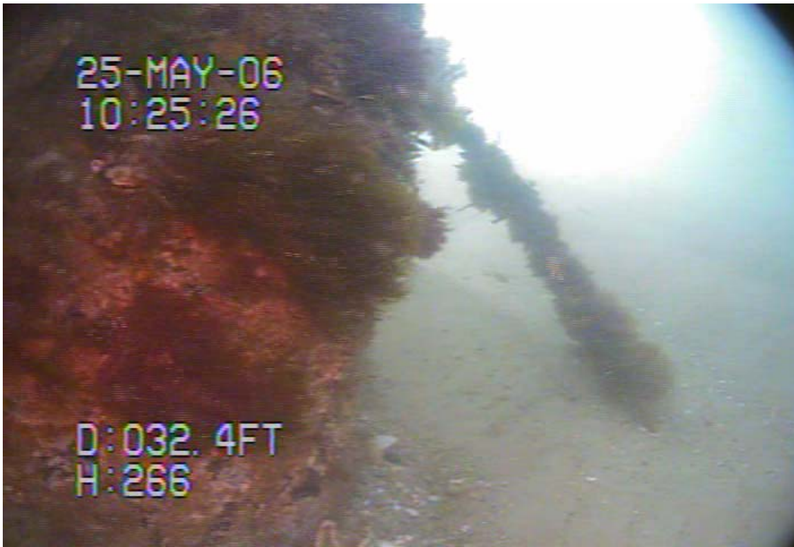
14. Scour at base of North pile
