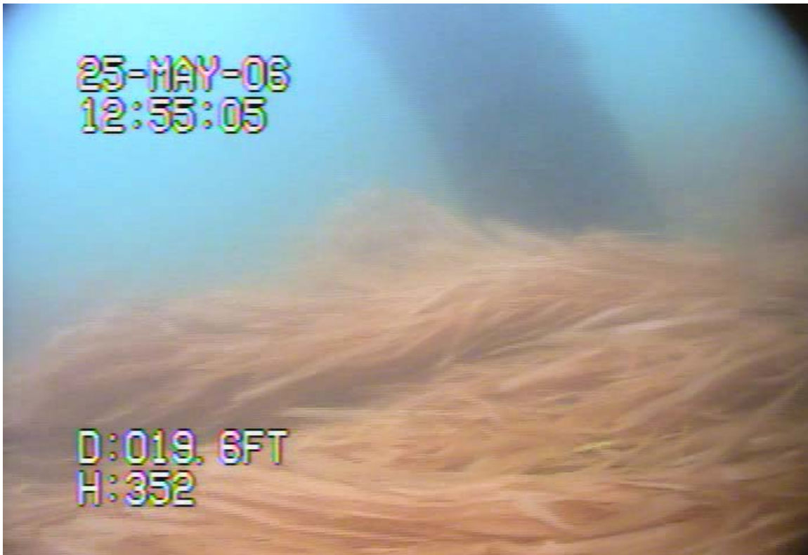
7. Newly installed mats at base of Southeast pile, Southeast pile in background
