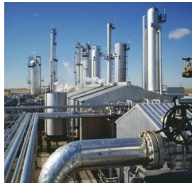
Natural Gas Processing
