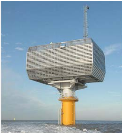
Figure 3. Offshore Power Substation. Source: https://www.jandenul.com/en/activities/offshore-services/offshore-wind-farms
