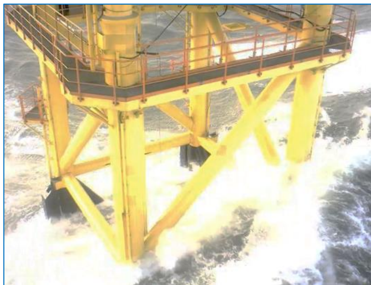
Breaking wave at FINO-1 platform in 28 m water depth when significant wave height is only 6 m
