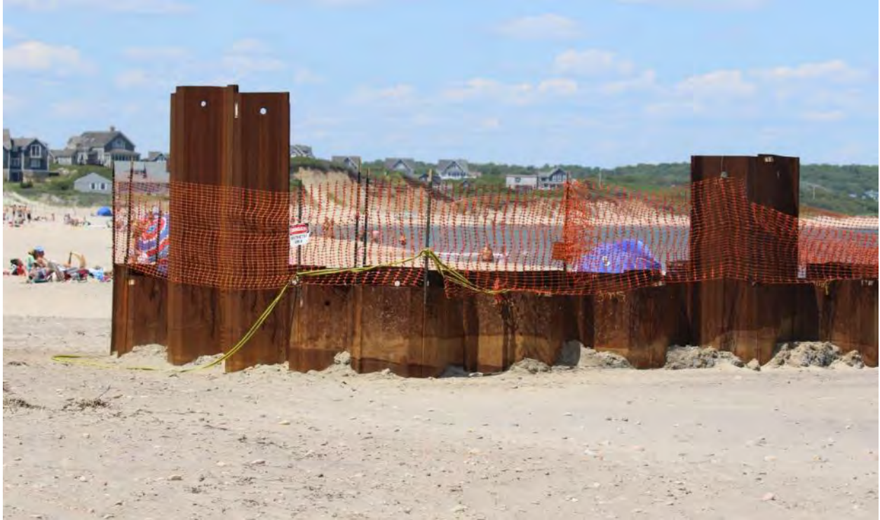
6/15/2016 Block Island Town Beach – Photo 3162: Close up of cofferdam prior to land sea transition.
