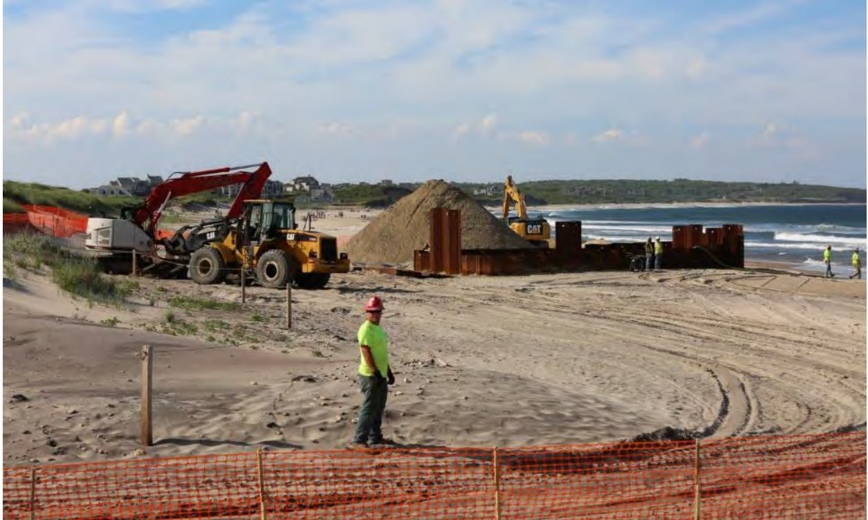
6/17/2016 Block Island Town Beach – Photo 0432: Crew preparing for land sea transition. Excavator removing sand from inside and in front of cofferdam.
