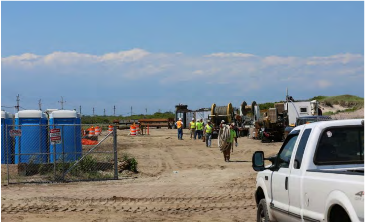
6/22/2016 Block Island Town Beach – Photo 0513: Construction area west of sand dune located north side of Fredrick J. Benson Pavilion adjacent to Corn Neck Road. Winch spool and winch visible used for pulling BITS to shore. Orange barrels surround land sea transition vault.
