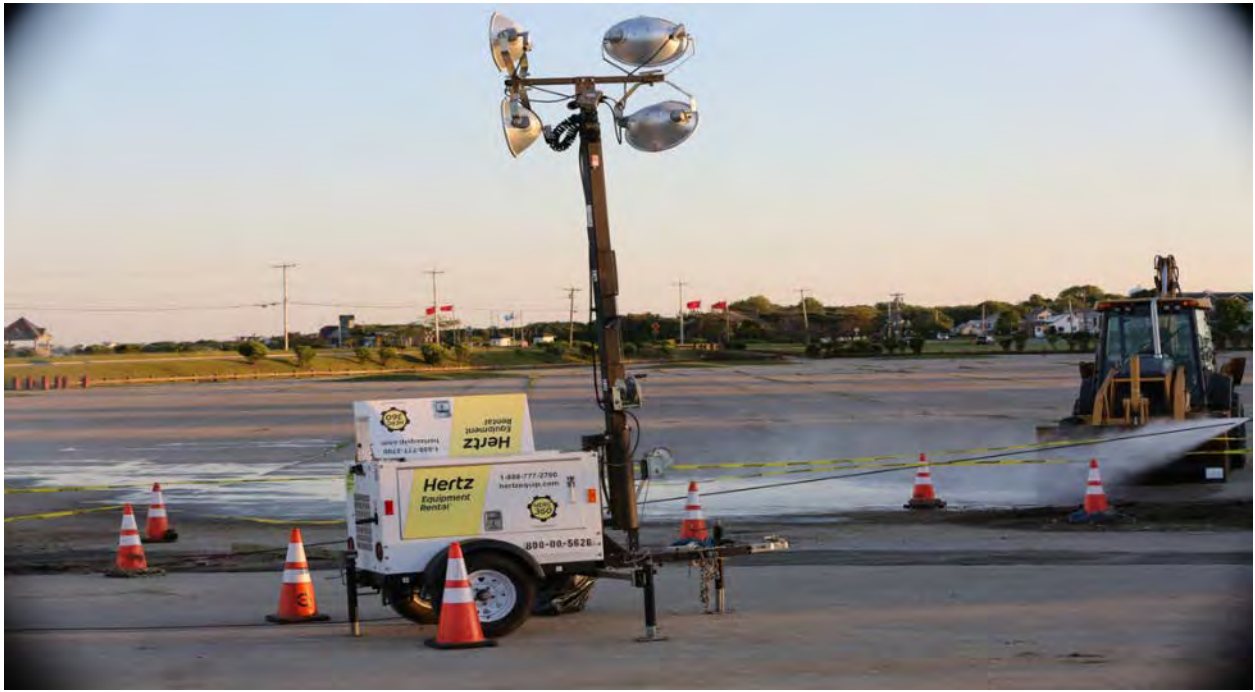
6/9/2016 Scarborough Beach State Park – Photo 0207: Portable lighting brought to site around dusk during cable pull. The winch cable is being washed as it is pulled back into shore.
