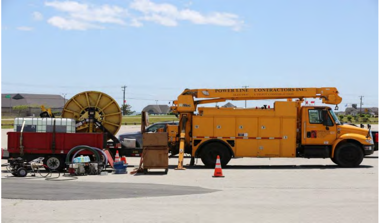
6/9/2016 Scarborough Beach State Park – Photo 0171: Cable pull initiation. Utility truck, winch spool, trailer with water and pressure washer used to spray salt water off the winch cable upon retrieval.
