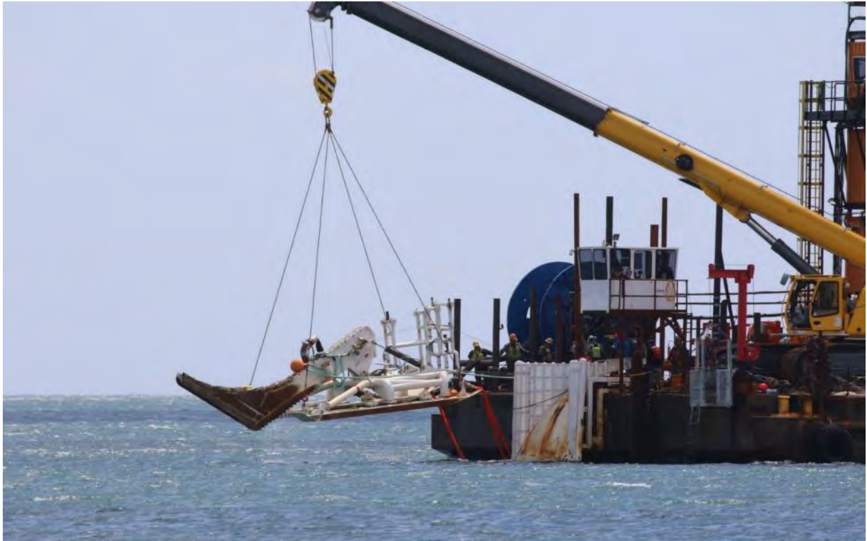
6/9/2016 Scarborough Beach State Park – Photo 2740: Jet Plow being lowered into the water aft of CLB Big Max.
