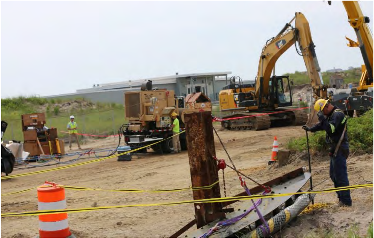
6/23/2016 Block Island Town Beach – Photo 0603: BITS cable pulled through land sea vault on north side of Fredrick J. Benson Pavilion adjacent to Corn Neck Road.
