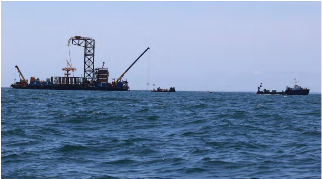
6/17/2016 Offshore – Photo 3348: CLB Big Max crossing CB-1 cable. Tender barge, dive tender, and support vessel Meghan Miller are supporting.
