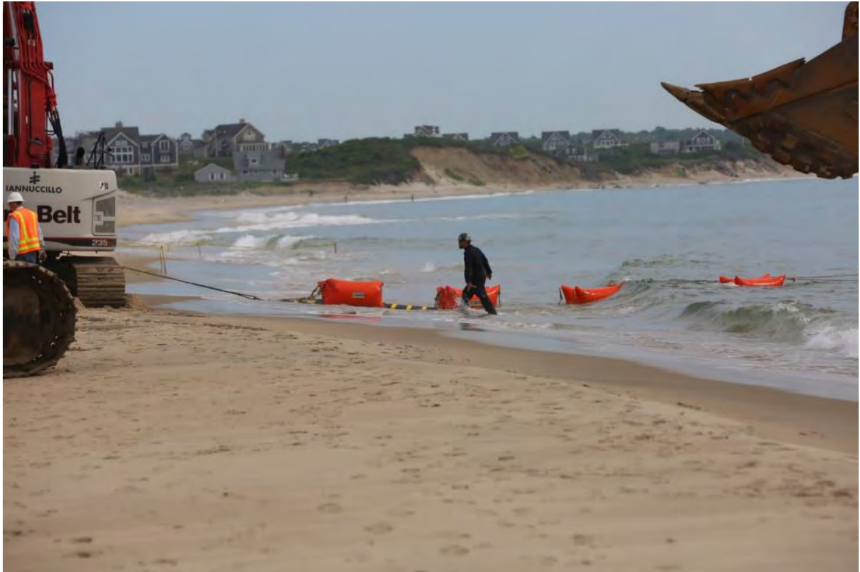
6/23/2016 Block Island Town Beach – Photo 0580: BITS cable coming ashore in front of cofferdam.
