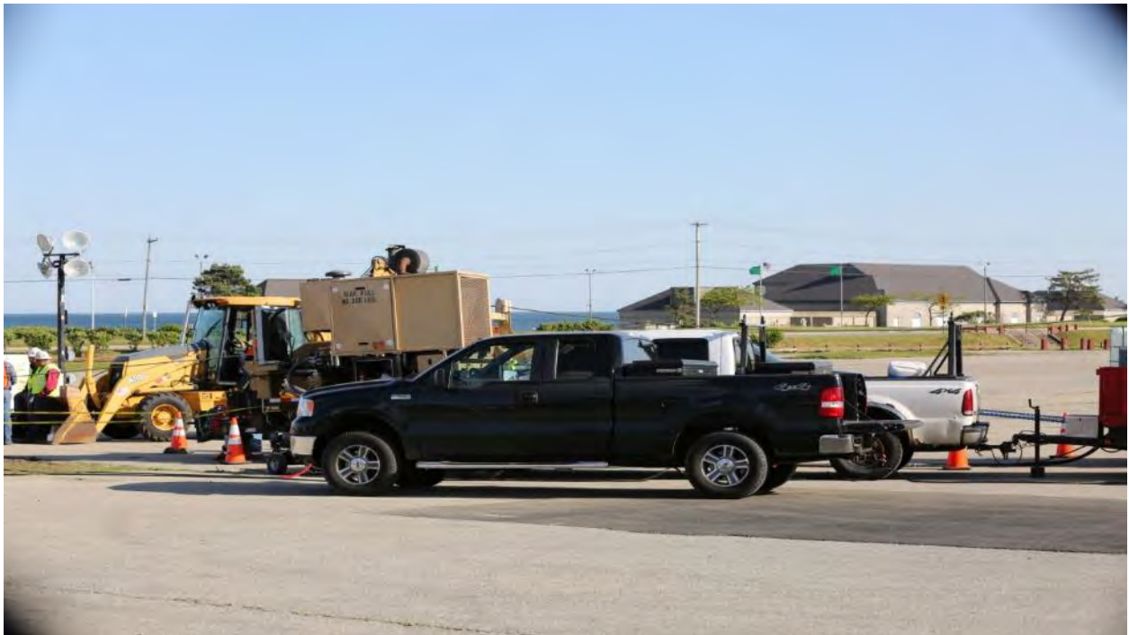
6/9/2016 Scarborough Beach State Park – Photo 0194: Trucks, winch, and backhoe located west of the land sea transition vault during cable pull.
