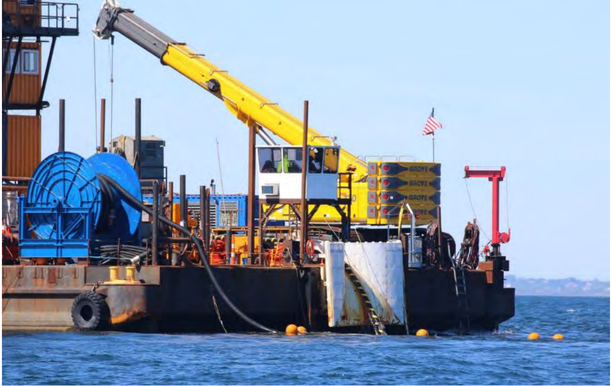
6/14/2016 Offshore – Photo 3009: BITS cable exiting chute on CLB Big Max and feed to jet plow.
