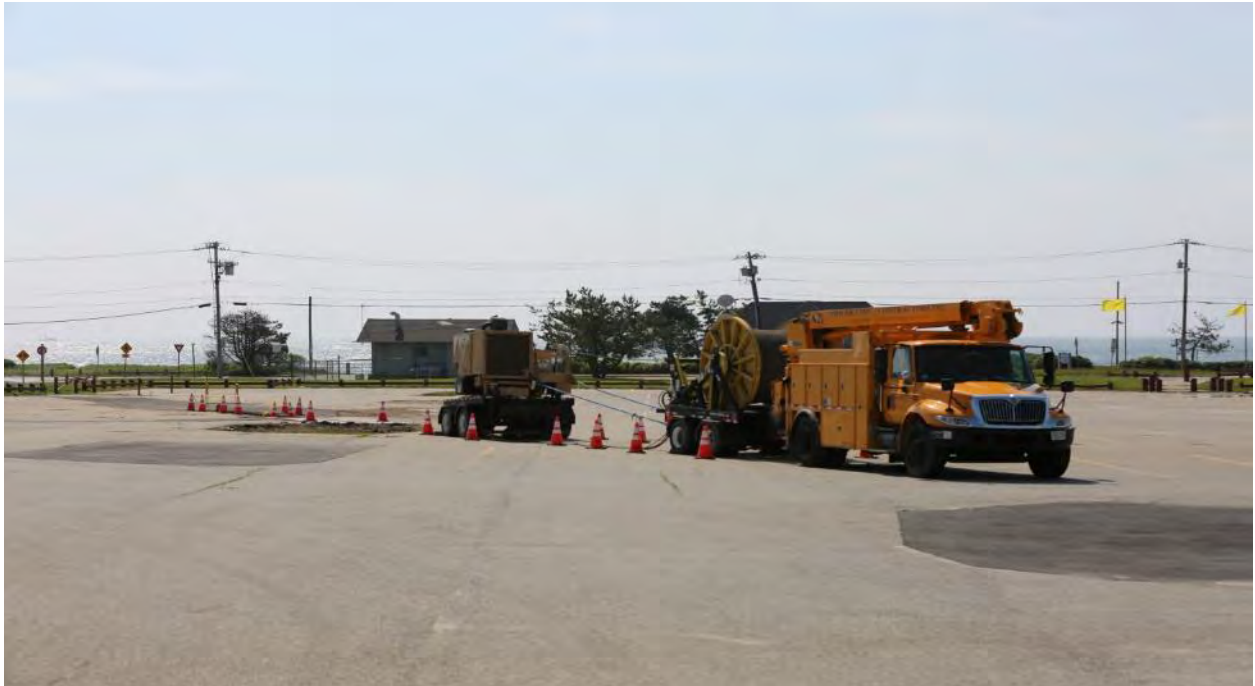
6/6/2016 Scarborough Beach State Park – Photo 0074: Utility truck, winch spool, and winch prepared for BITS cable pull to shore. The land sea transition vault is surrounded by cones.
