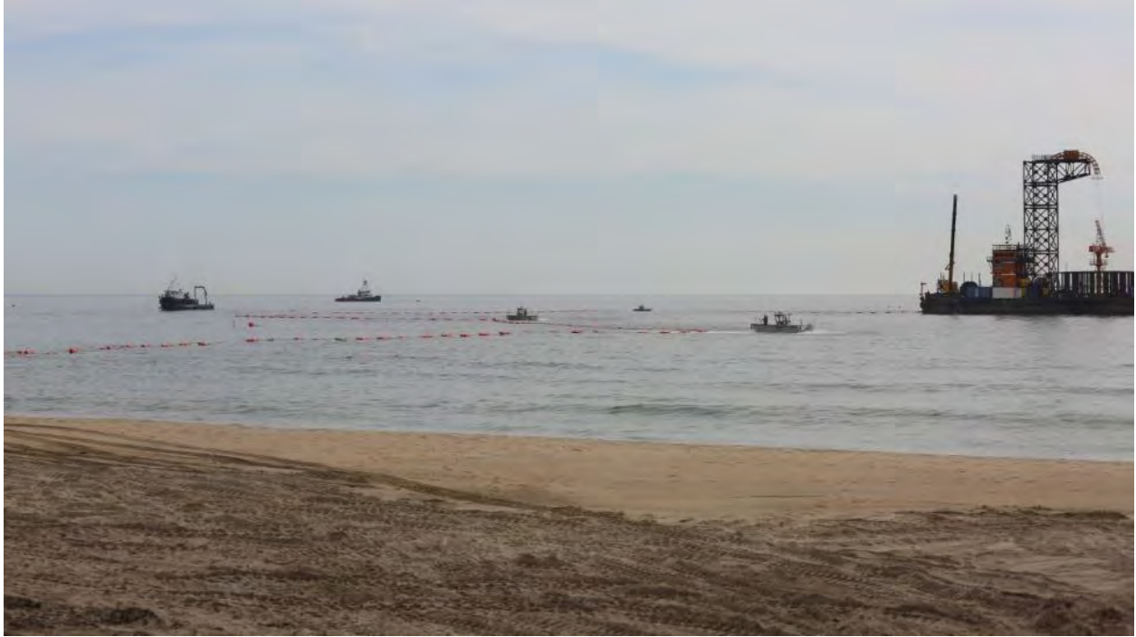
6/23/2016 Block Island Town Beach – Photo 0570: “Floating the cable”, orange buoys floating the remaining BITS cable to the surface in preparation for pulling to shore.
