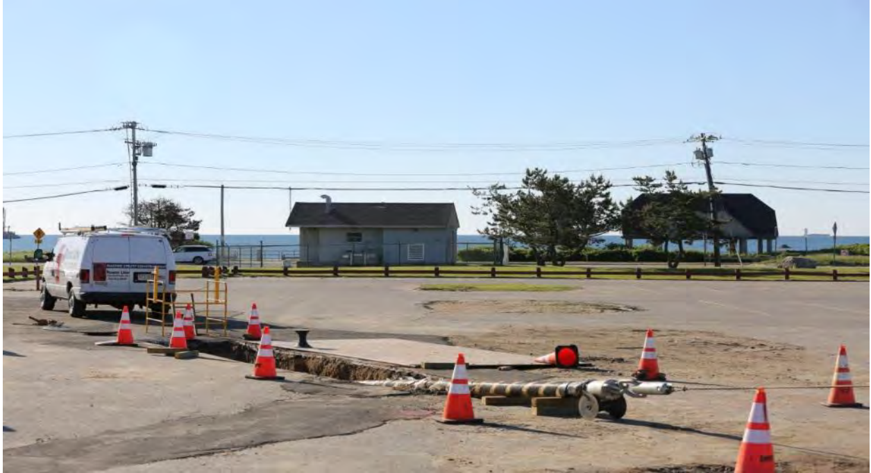
6/10/2016 Scarborough Beach State Park – Photo 0207: BITS cable attached to winch cable at the land sea transition vault.
