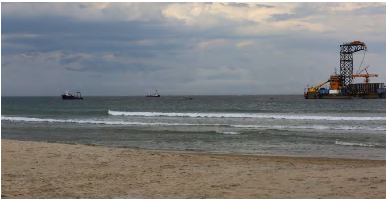
6/22/2016 Onshore – Photo 0522: Messenger cable was pulled of CLB Big Max, orange buoys were attached by divers and used to float messenger cable. The messenger cable is then connected to onshore cable winch which is pulled back to CLB Big Mad. The cable winch is used to pull BITS to shore. Support vessels Joel Miller and Meghan Miller visible.
