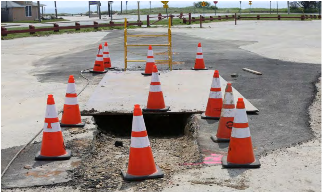
6/7/2016 Scarborough Beach State Park – Photo 0106: Land Sea Transition Vault prior to cable pull.
