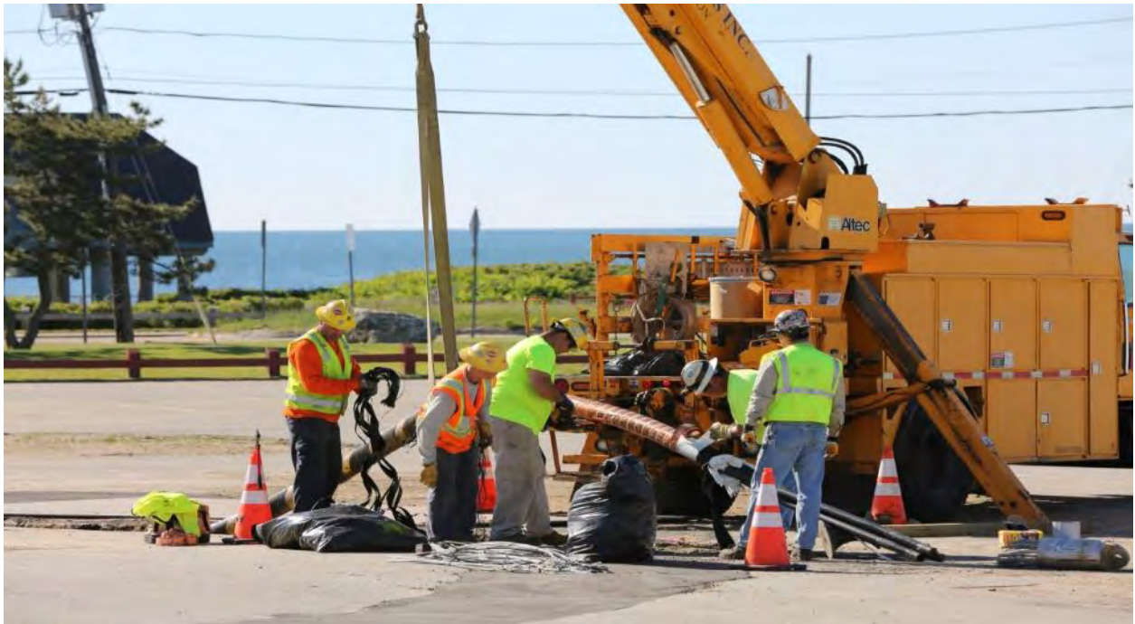
6/10/2016 Scarborough Beach State Park-Photo 0252: Stripping outer casing of BITS cable in order to splice into terrestrial cable.
