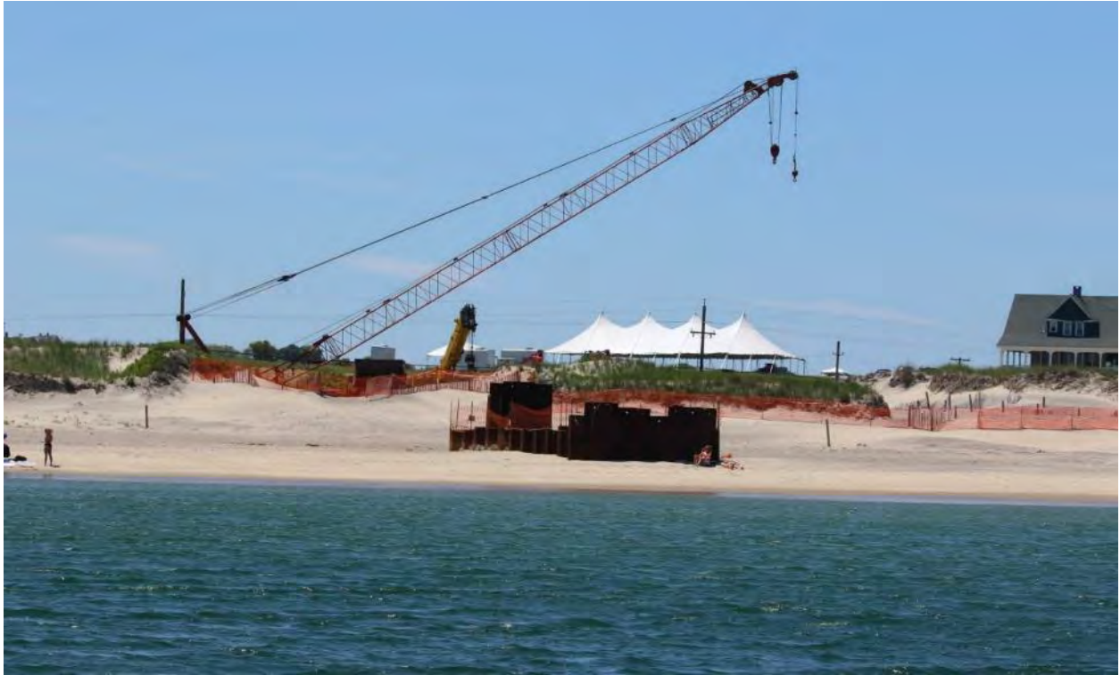
6/15/2016 Block Island Town Beach – Photo 3156: Cofferdam prior to arrival of CLB Big Max. Construction equipment parked behind sand dune.
