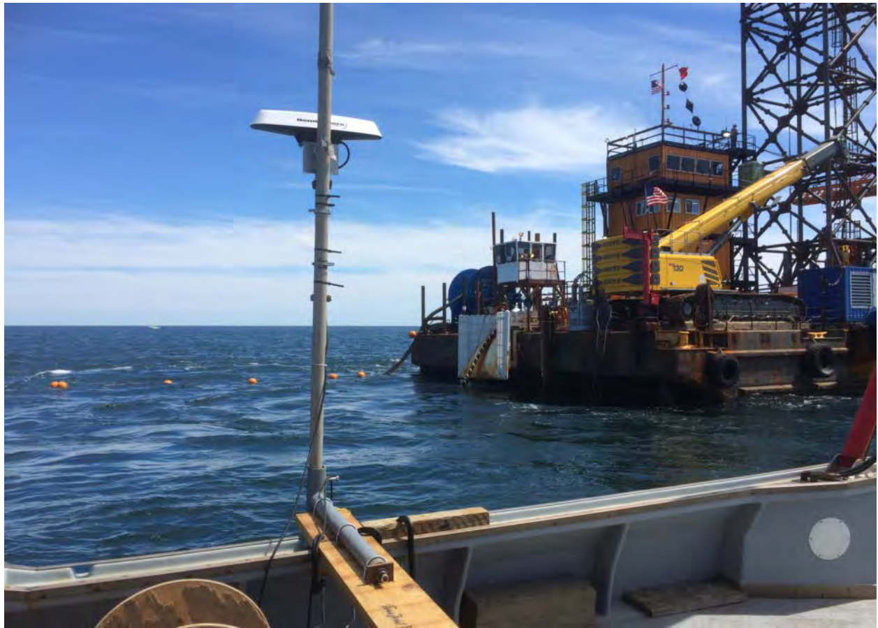
Figure 18. ADCP and DGPS installed on a pivoting arm aboard the Jamie Hanna with the cable lay vessel Big Max and buoys marking the jet plow in the background
