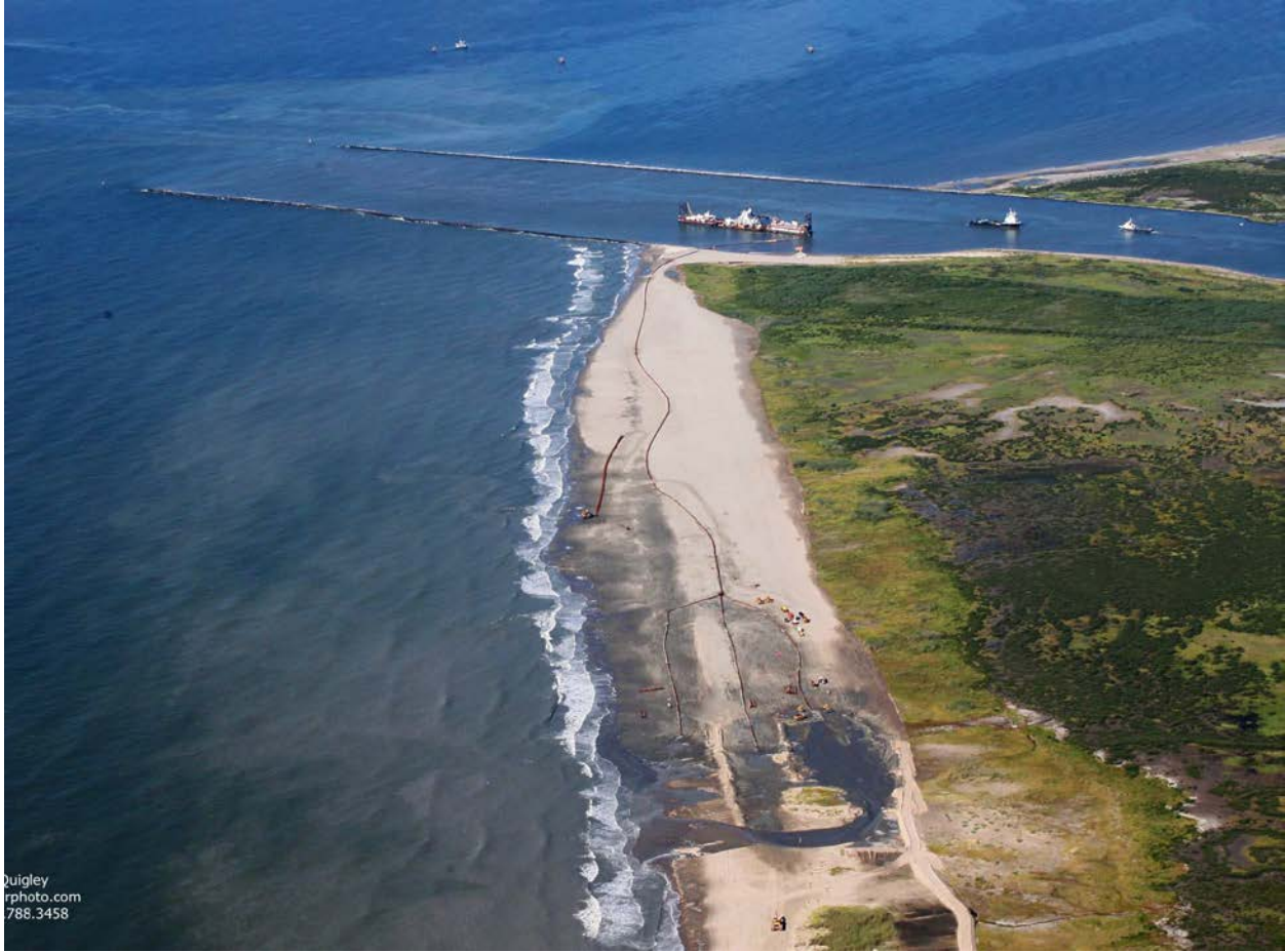
Figure 8. Aerial photograph of Caminada Headland construction, September 6, 2013. Photo credit: Patrick M. Quigley ( www.gulfcoastairphoto.com ).
