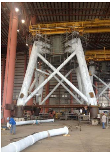
Fabrication of Block Island Foundations by Gulf Island Fabricators, in Houma, LA
