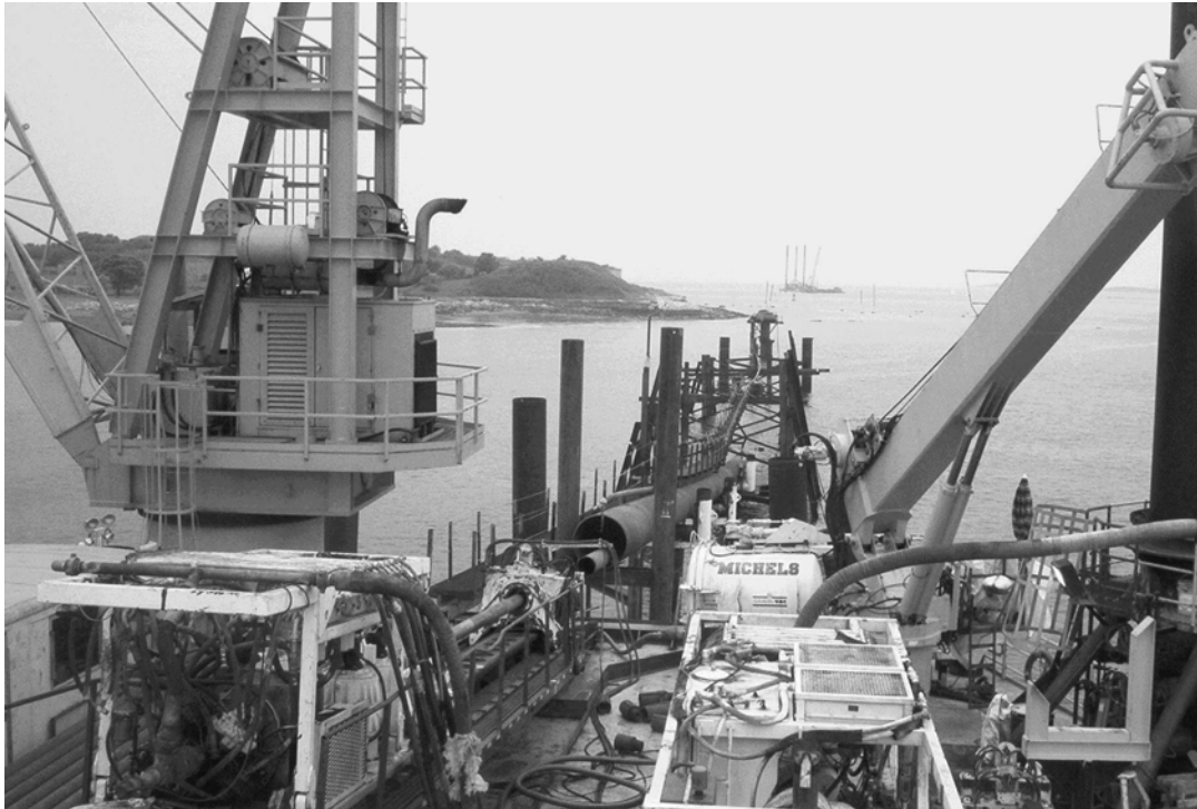
Figure 3 - Marine Riser at Georges Island
