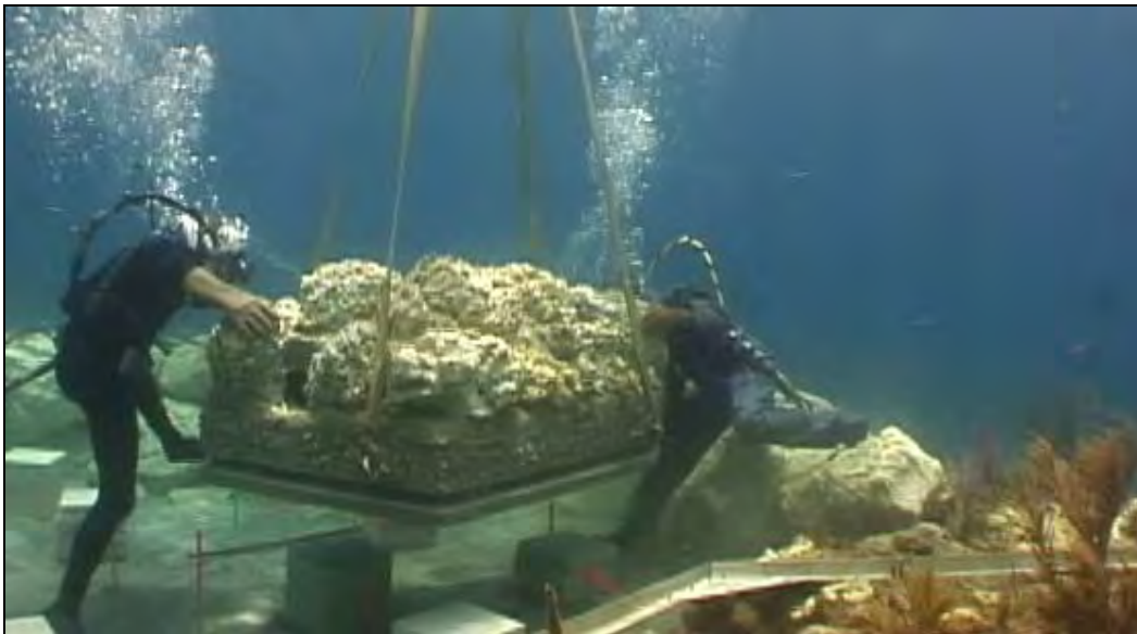
Figure 12 Habitat Replacement Module Deployment Requiring Commercial Dive Operations and Marine Operation Heavy Equipment
