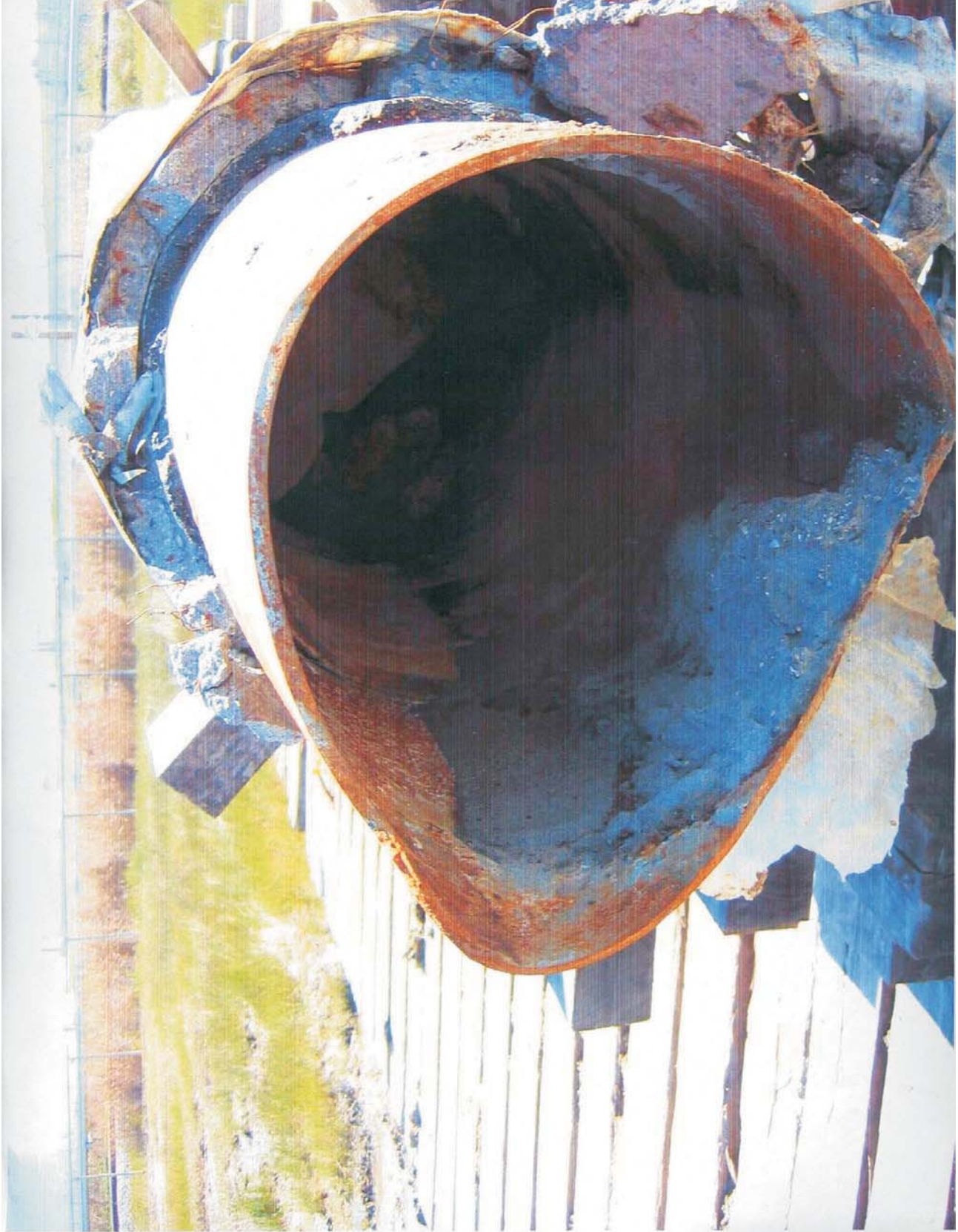
Photograph of pipeline break – impact detail
