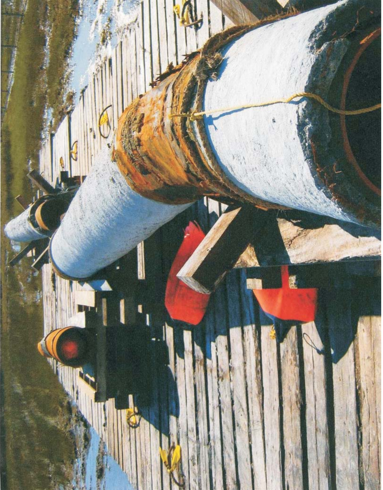
Photograph of pipeline break – platform side
