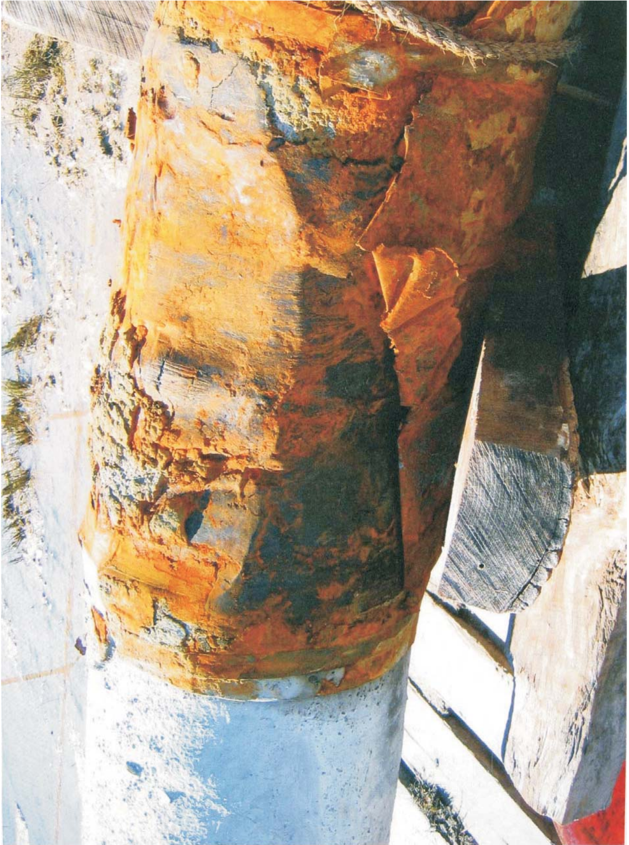
Photograph of pipeline concrete coating impact
