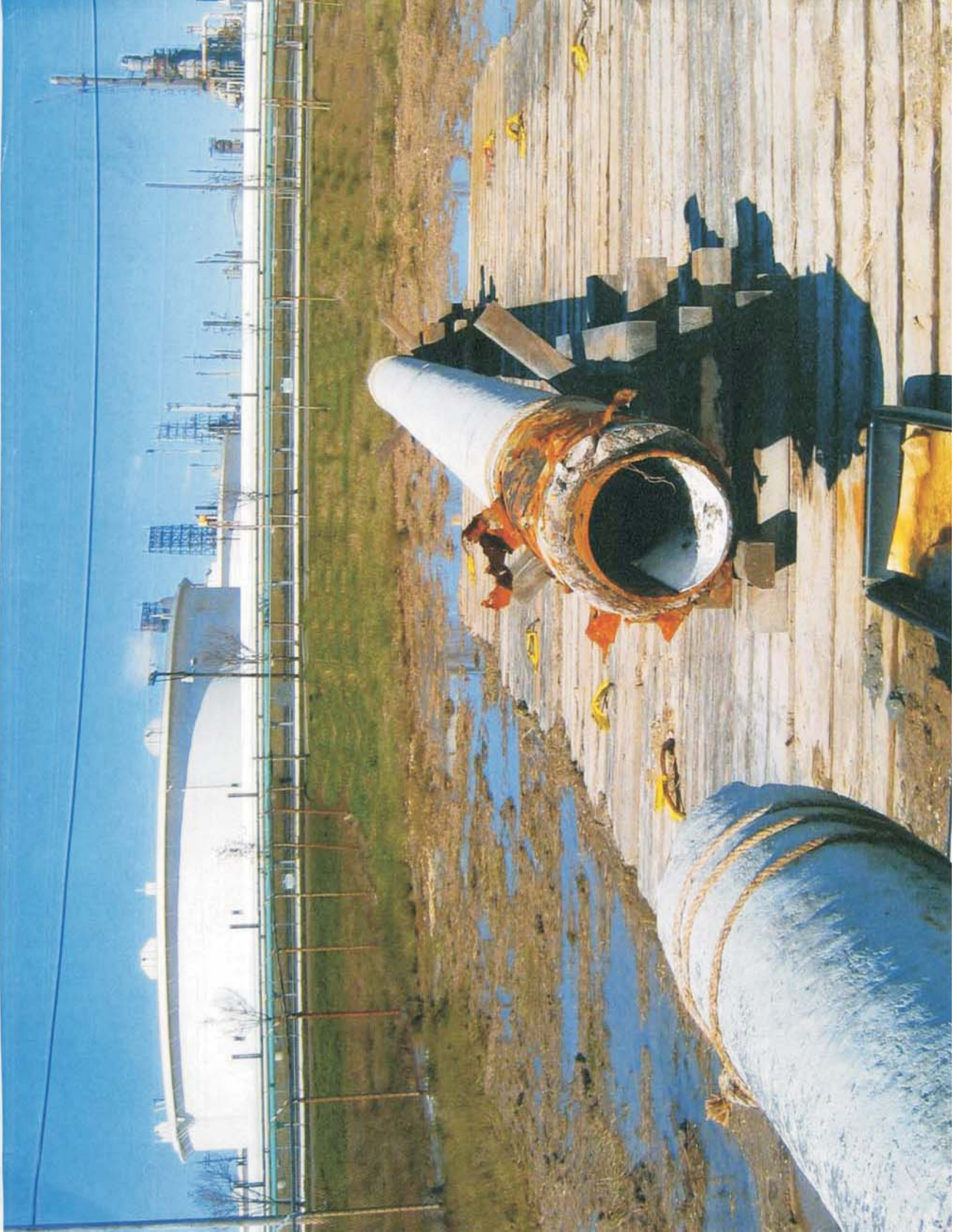
Photograph of pipeline break – shore side
