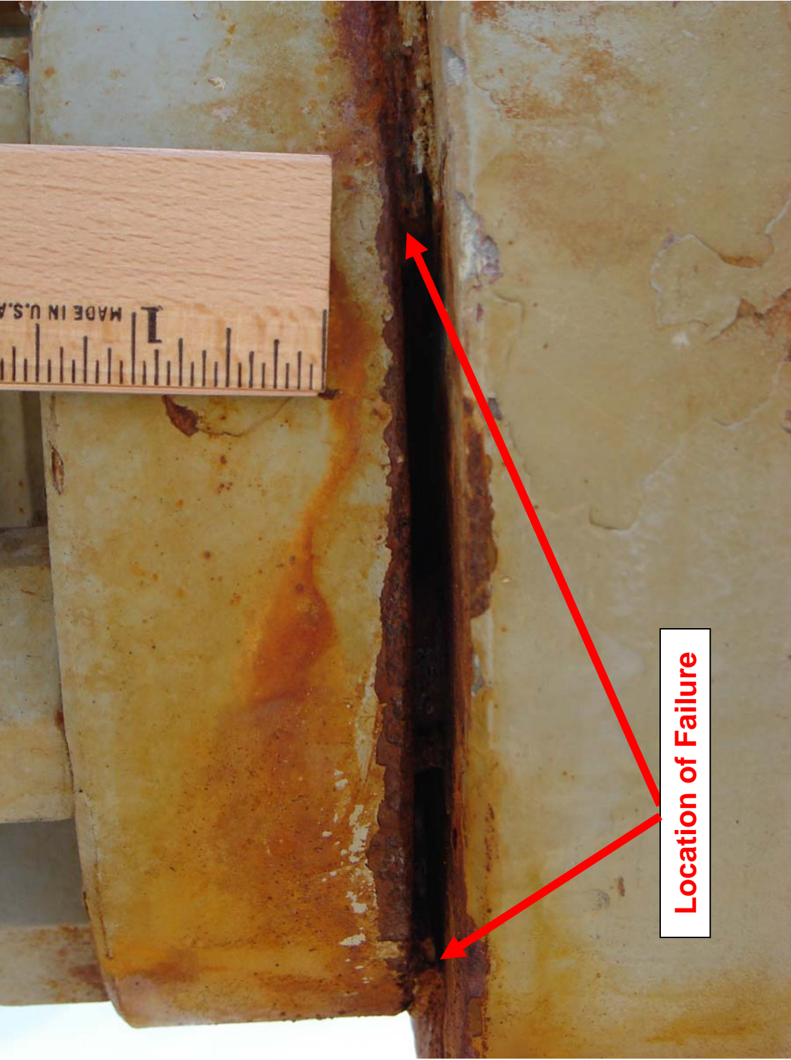
Photo of Connection Between Master Valve and Adapter Flange (Location of Ring Gasket Failure)
