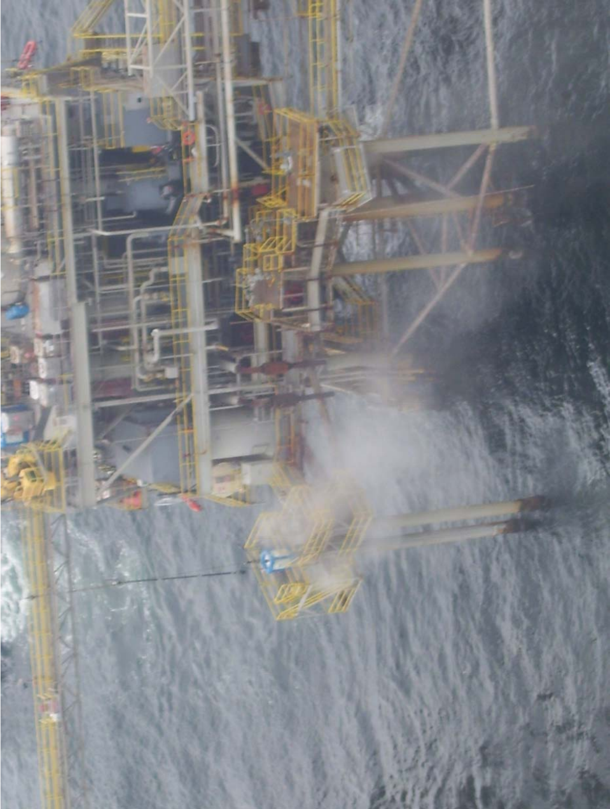
Photo of PL 10 During Loss of Well Control
