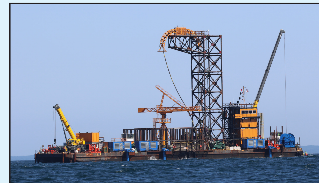
Cable lay vessel.
