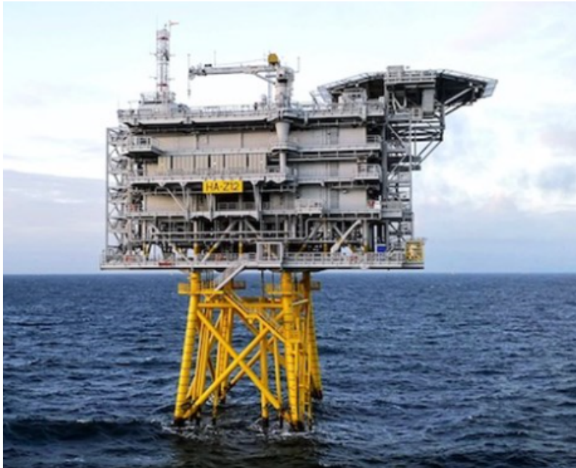
Figure 6.1.1-7. Indicative offshore substation with helideck (Hornsea I).
