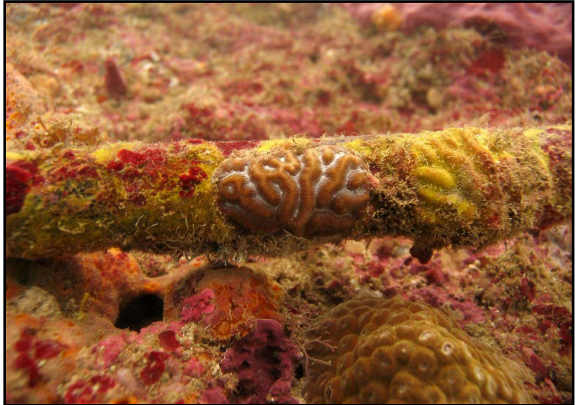
Telecommunications cable with encrusting marine organisms
