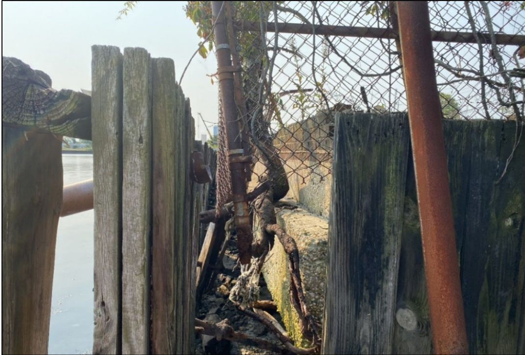
Figure 2.2-4. Close up of bulkhead in disrepair, showing thick concrete foundation pad and remains of a brick wall.
