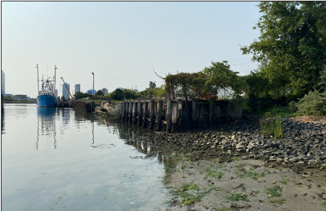
Figure 2.2-3. Overview of partially collapsed wood and concrete bulkhead facing the marina. View to the south.
