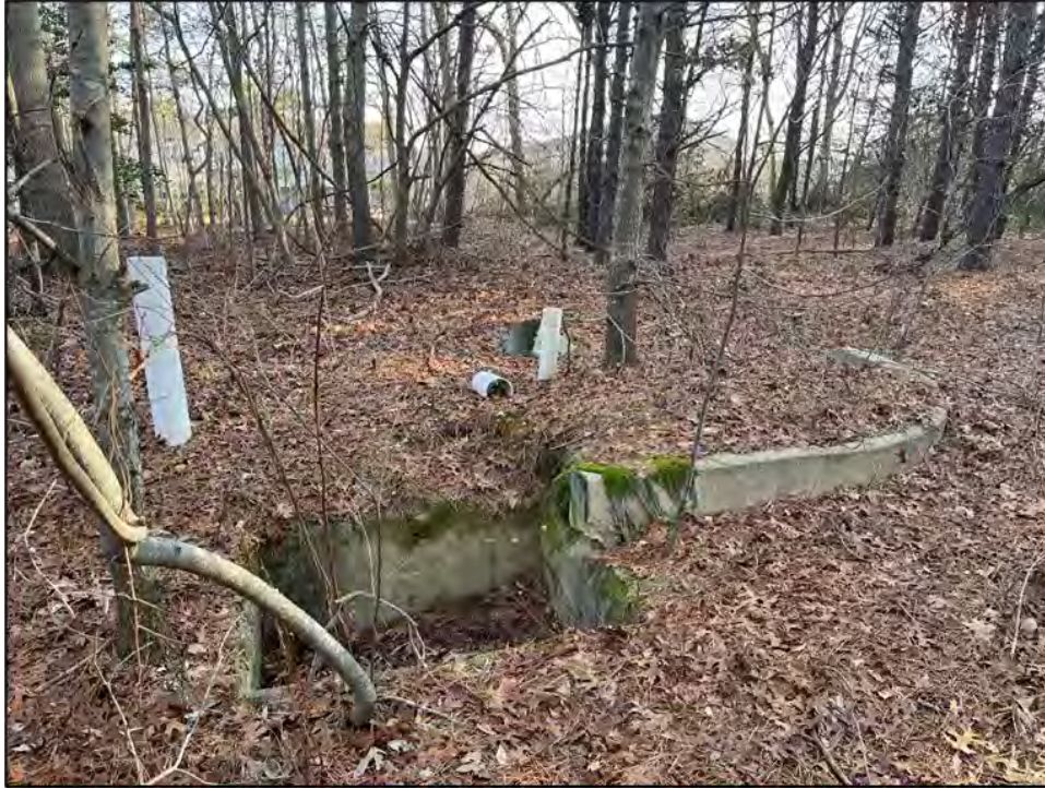
Photograph 36. Detail of storm drain and curbs along the access road. An excavation trench can be seen in the background to the right of the photograph, view to the east.
