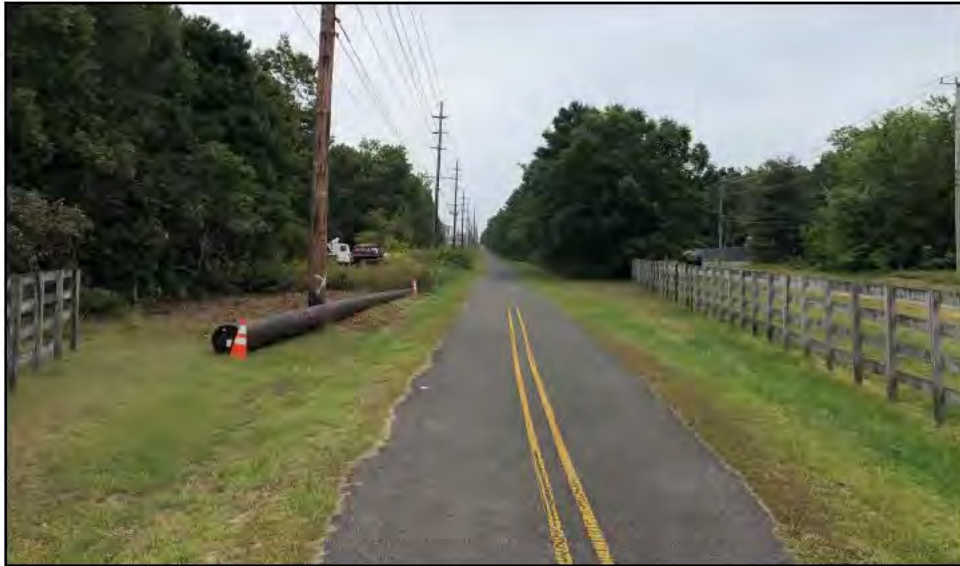
Photograph 30. Overview of the Cardiff Onshore Route at the intersection of Winter Green Avenue and the Atlantic County Bikeway along the former West Jersey Railroad corridor. View to the southeast.
