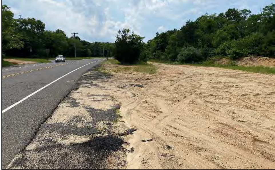
Photograph 9. View of HDD pit exit area along Lakewood-Allenwood Road, with heavy surface disturbance and soil push piles on mapped sand and gravel pits. View to the west.
