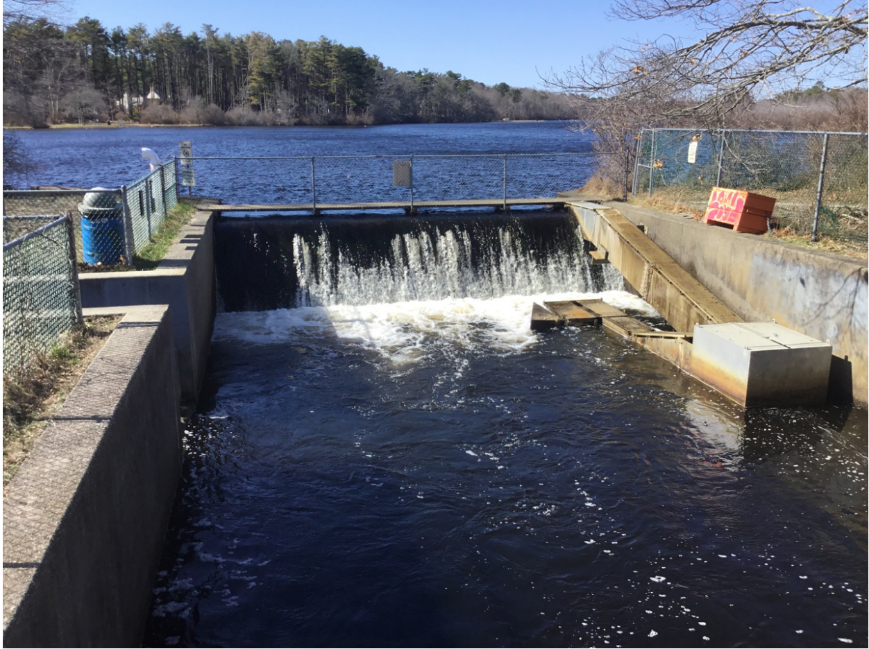
Photograph 18. Watercourse S-01GP. View northwest of Dam on Carmans River from Victory Avenue. Stantec. March 2021.
