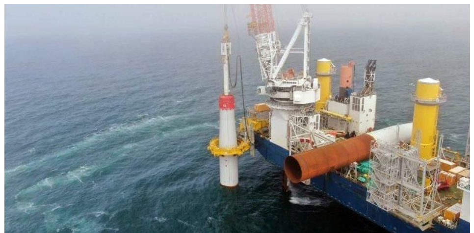
Photo: Double bubble curtain around a monopile foundation during installation at CVOW.
