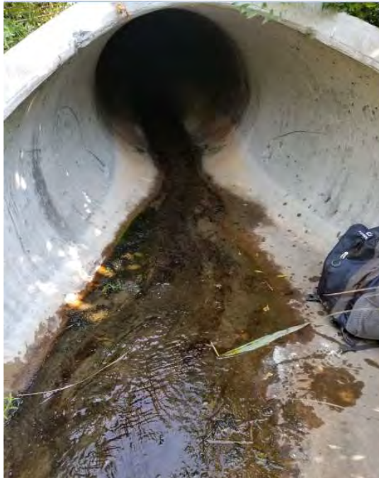
Photo 4: Concrete outfall pipe from the Confined Disposal Facility east of Route 9. Pipe widens to a six-foot wide splash pad; area immediately below splash pad is flooded at high tide.
