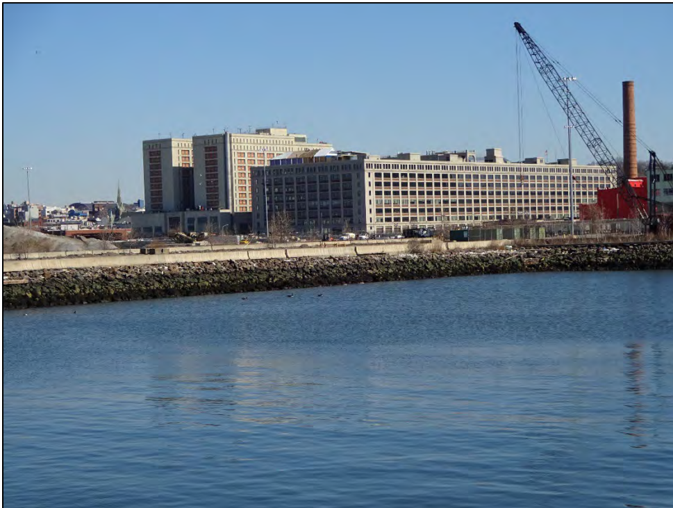
Close-up of Storehouse No. 2 from 39 th Street "Pier" at SBMT. "Interpier" basin will be dredged and new paving and structures will be installed on the "pier".
