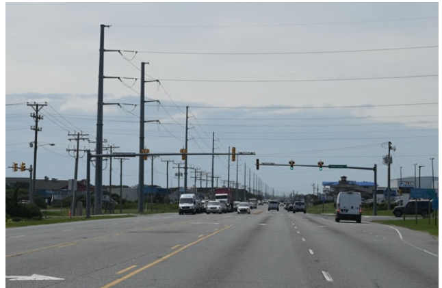
Transmission lines paralleling Route 158 in Kitty Hawk.
