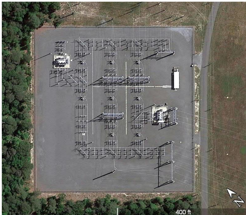
Figure 2-19. Indian River Substation
