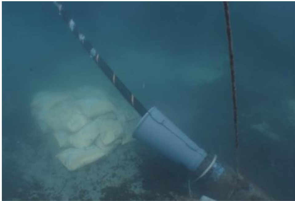
Figure 3-9. Underwater View of Near Shore Cable Pull into HDD Duct Source: Nexans.com
