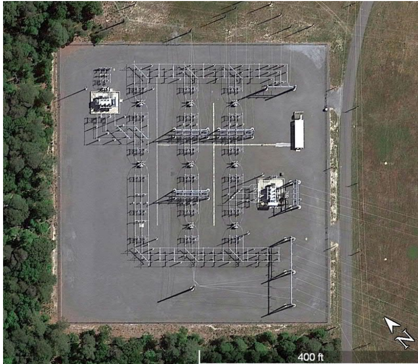
Figure 2-20. Indian River Substation
