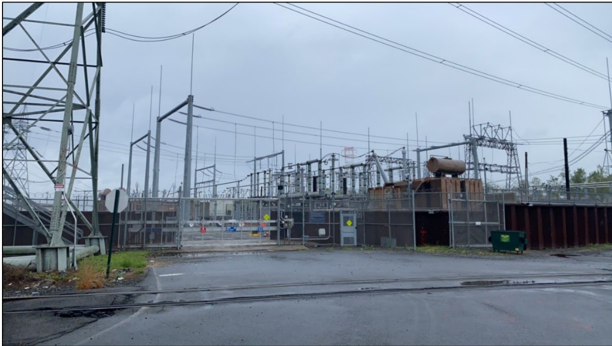
Figure 2.2-4. Overview of the existing Goethals Substation POI near the potential River Road Substation and/or Converter Station. View to the northeast.
