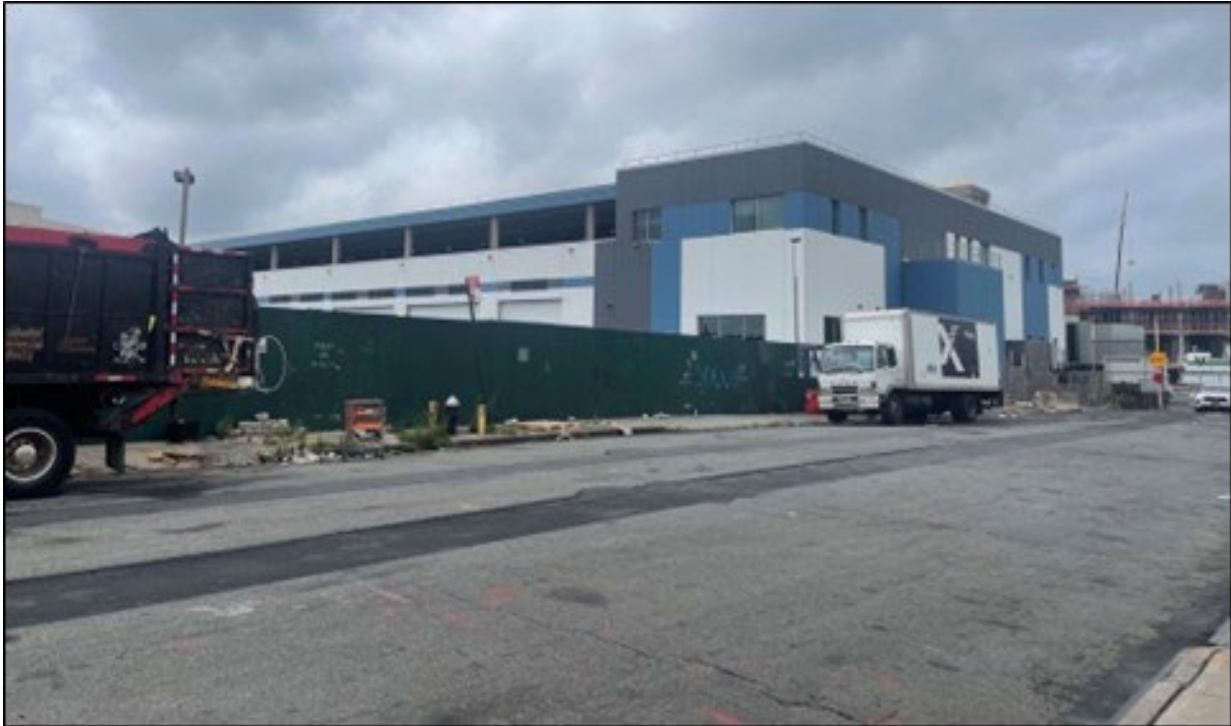
Figure 2.2-5. Overview of the new and active construction occurring at Sunset Industrial Park Onshore Substation and/or Converter Station Site, from public right-of-way on 19 th Street. View to the west.
