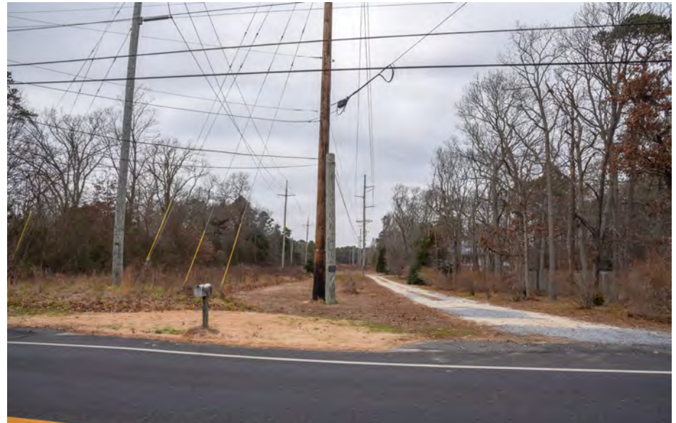
303 Upper Township - Proposed Underground Cable Route to BL England, Old Tuckahoe Road N
