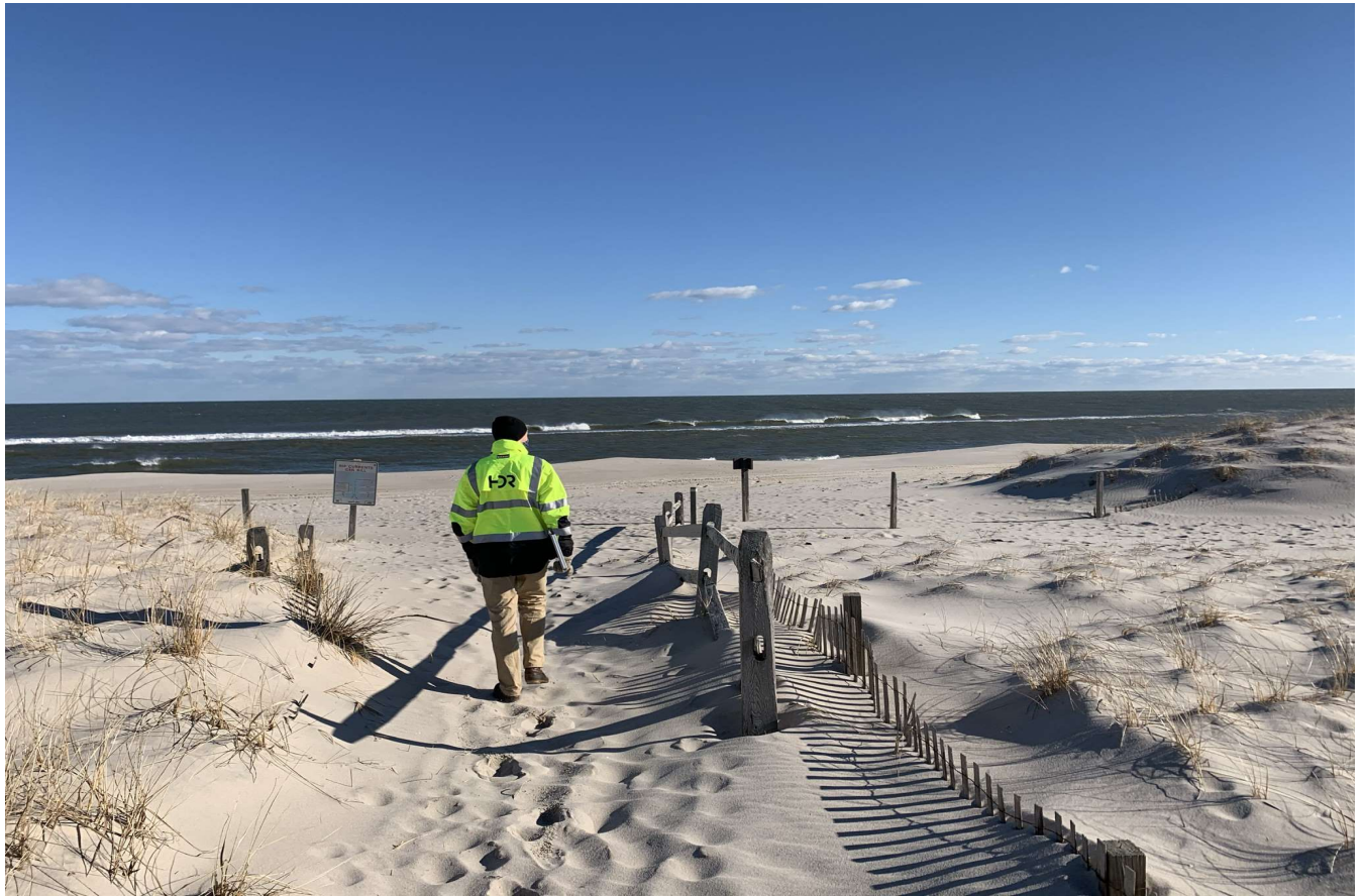
Photo 21: Viewing east at Atlantic Ocean from Island Beach State Park dune beach access path, area of HDD exit pit in the distance
