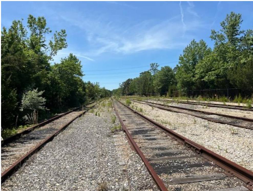
Photo 6 – Edge of railroad tracks on the southeast corner of the review area, viewing south.
