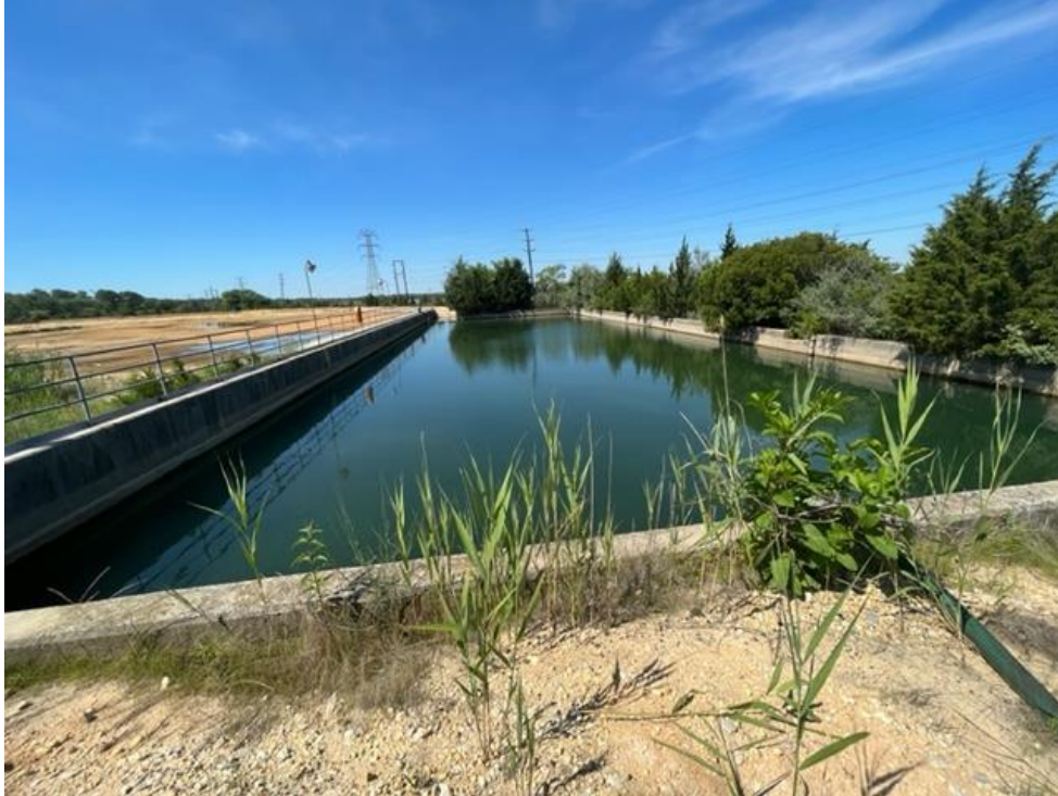
Photo 1 – Concrete lagoon on northern end of the review area. Water clear; about four feet deep.
