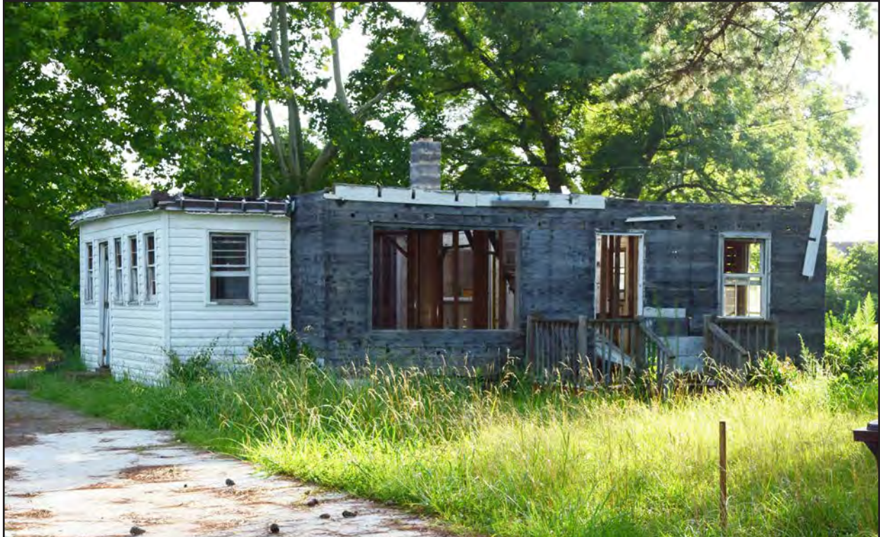
Figure 34. 131-5982, remnant of Minimal Traditional dwelling, southwest and northwest elevations, view to the east.
