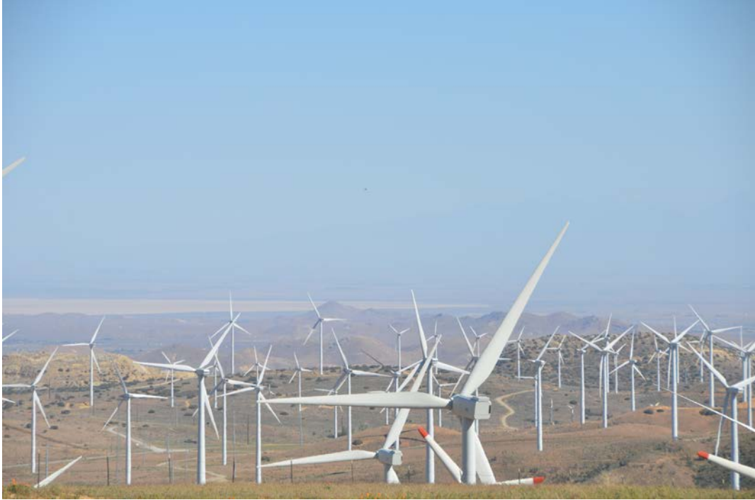
Figure 4. Wind Turbines at the TWRA
