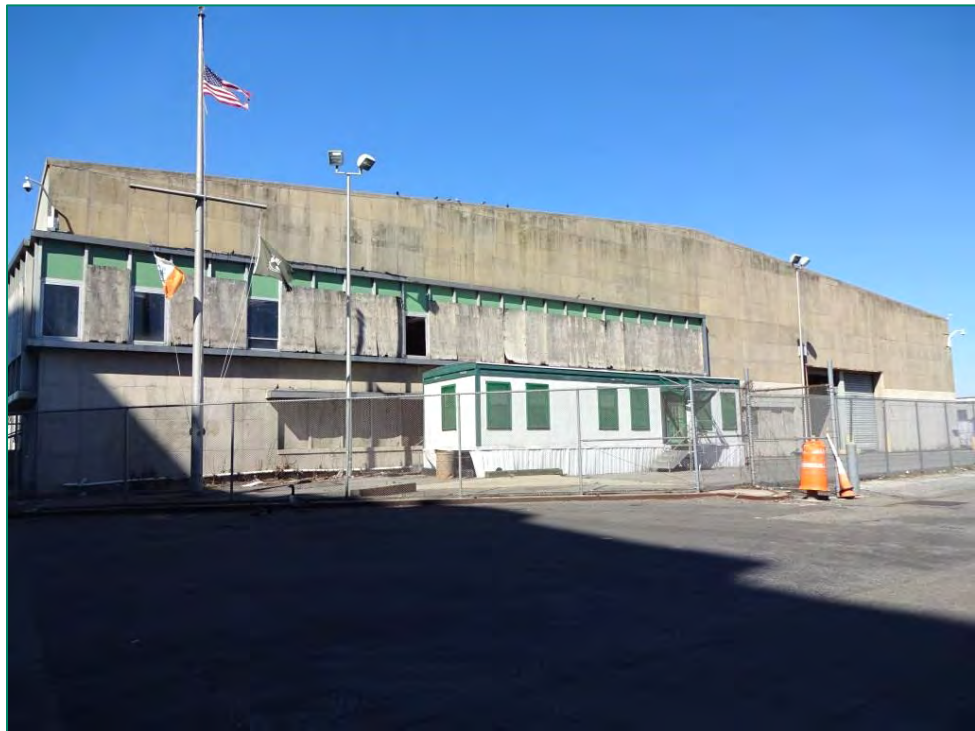
Looking northwest toward existing building structure at SBMT (39th Street "Pier"); structure will be removed.
