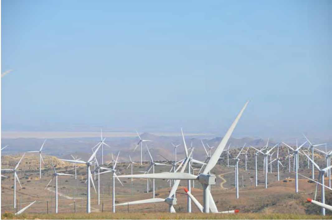
Figure 4. Wind Turbines at the TWRA
