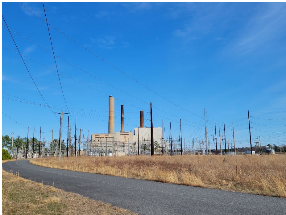
Figure 2-4. NRG Indian River Power Plant
