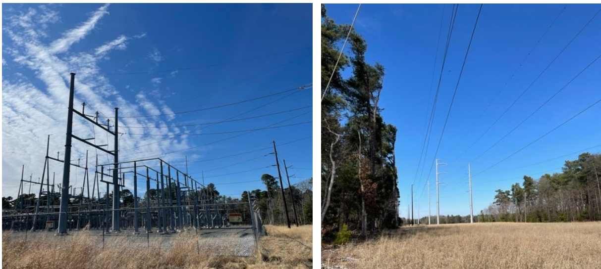
Figure 2-2. Existing Indian River Substation in Millsboro, Delaware
