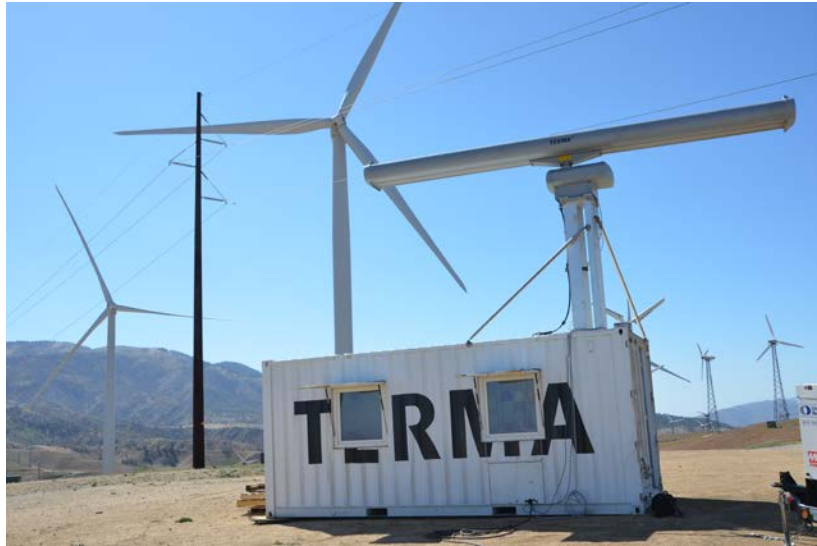
Figure 6. Terma SCANTER 5202 PSR Installed at TWRA
